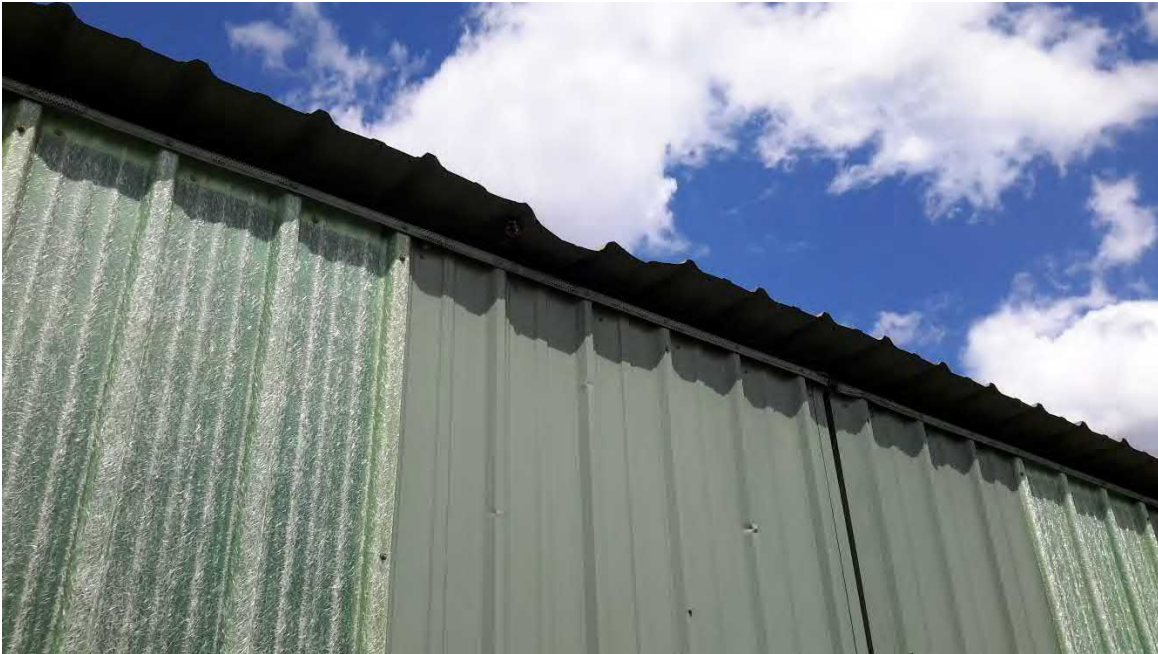
Figure 126 Hangar K - east side eave damage from snow and ice
