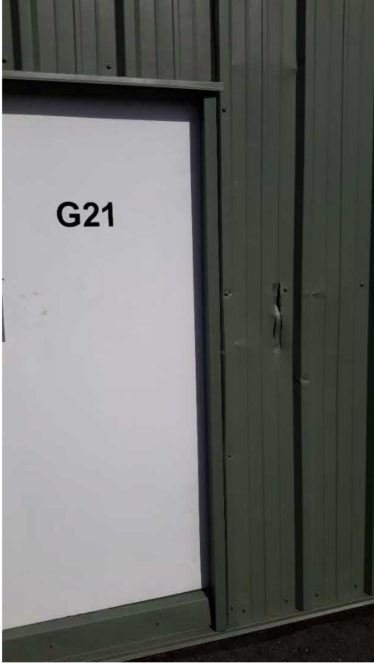
Figure 105 Hangar G - door panel damage (G21)
