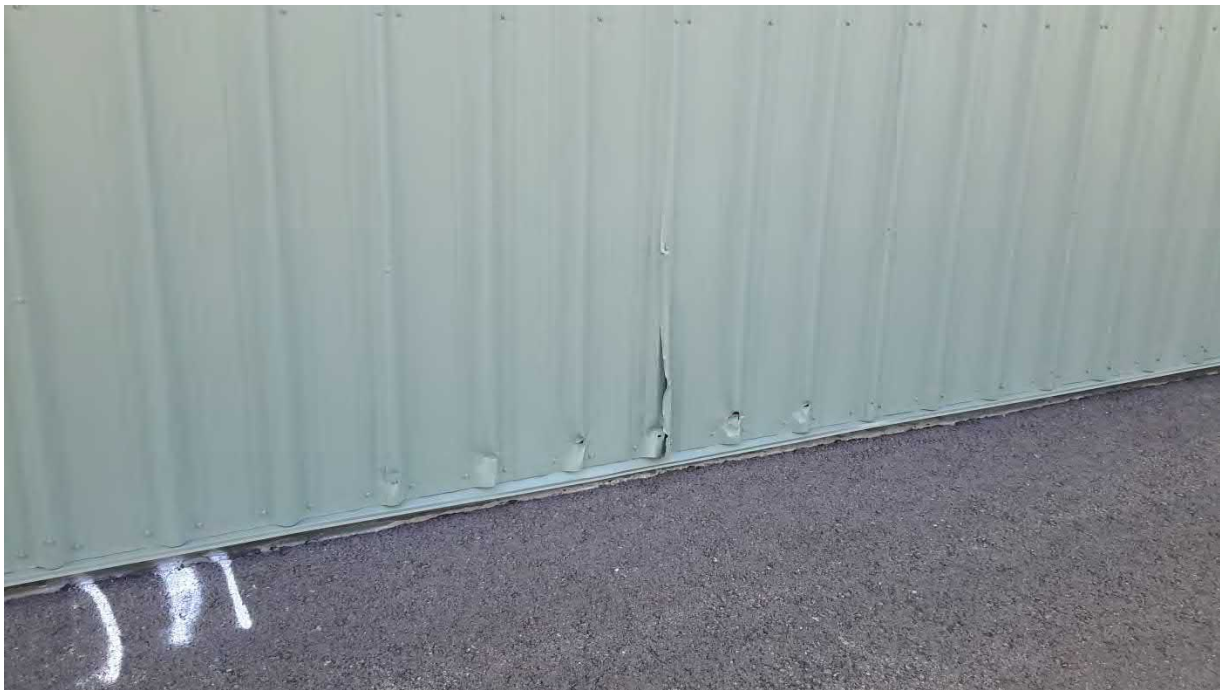
Figure 99 Hangar A - door panel damage (F2)
