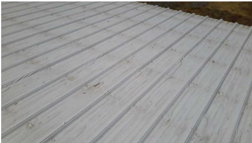
Figure 28 Building 11 - roof coating delamination
