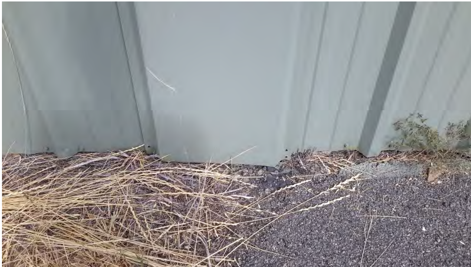
Figure 41 Building 12 - wall panel fasteners missing at base, east side
