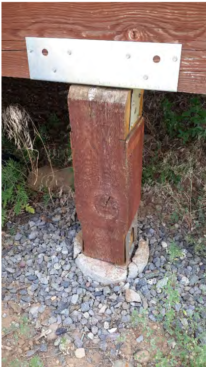
Figure 23 Building 9 - deck pier cracked and failing
