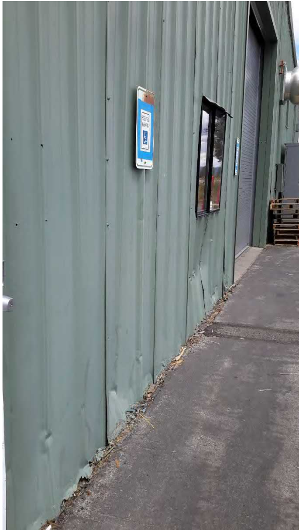
Figure 36 Building 11 - wall panel damage on east side from snow, ice and/or vehicles
