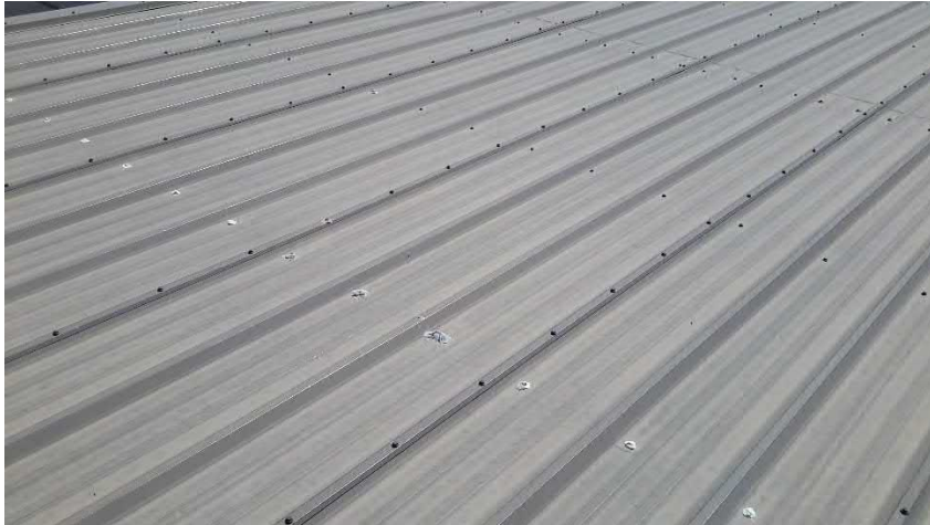
Figure 96 Hangar F - roof panels show crimping and kinking damage from snow and ice
