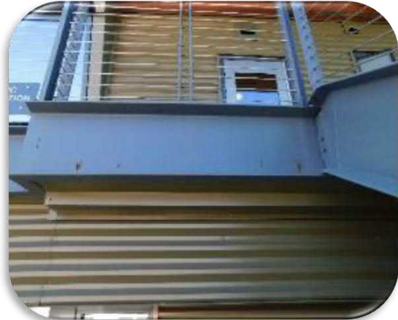
Figure 5-7 shows some minor spot rusting on the structural members.
