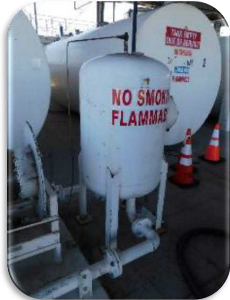
Figure 5-44 shows a view of the far end of the equipment skid with rust and impact damage.
