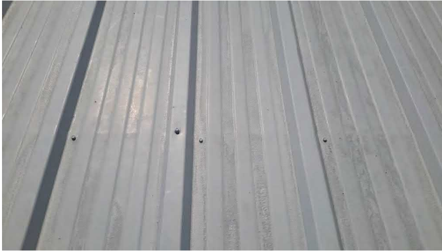
Figure 61 Hangar B - roof was coated over older screws some missing washers
