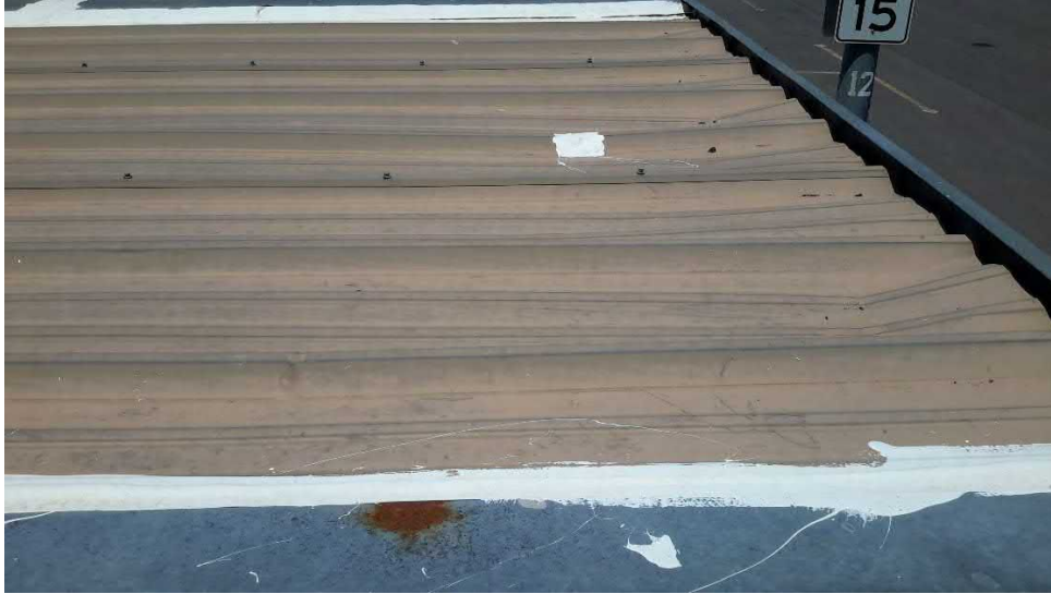
Figure 40 Building 12 - roof damage from snow and ice
