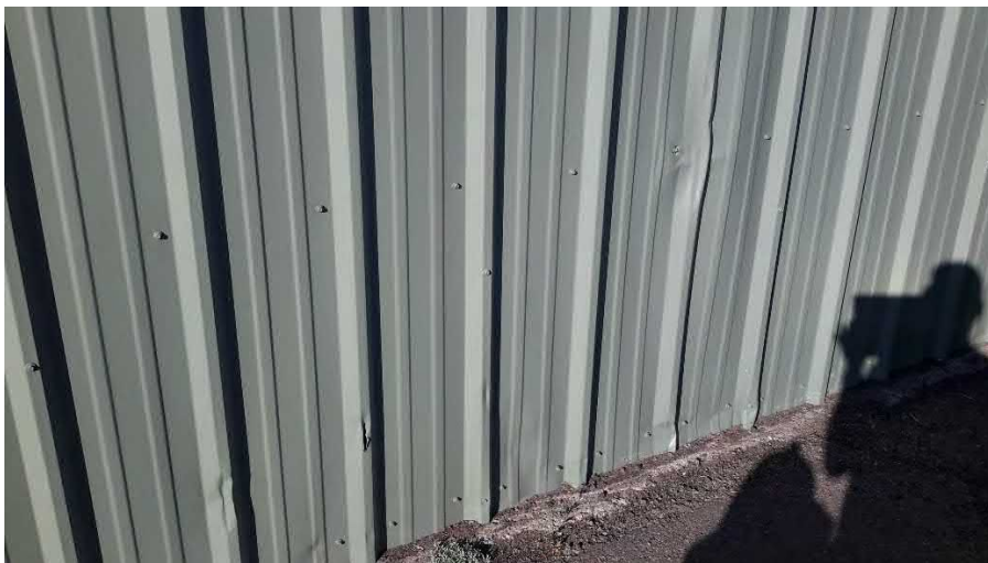
Figure 57 Hangar A - wall panel damage on north end
