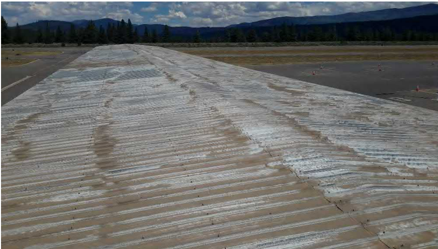
Figure 117 Hangar J - roof panel paint coat badly worn
