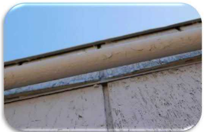
Figure 5-60 shows the condition of the piping associated with the EAA Building.
