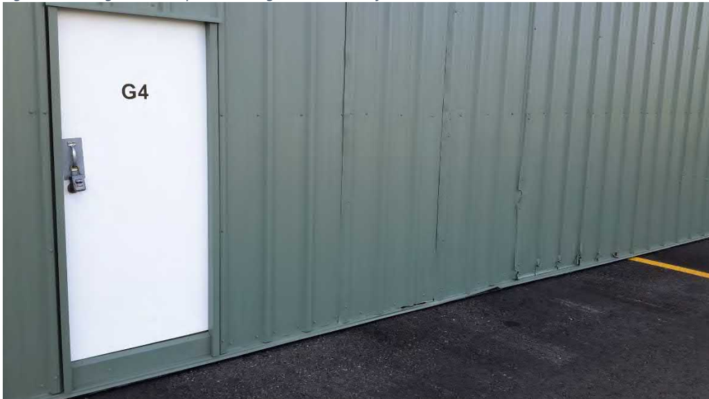
Figure 104 Hangar G - door panel damage (G4)
