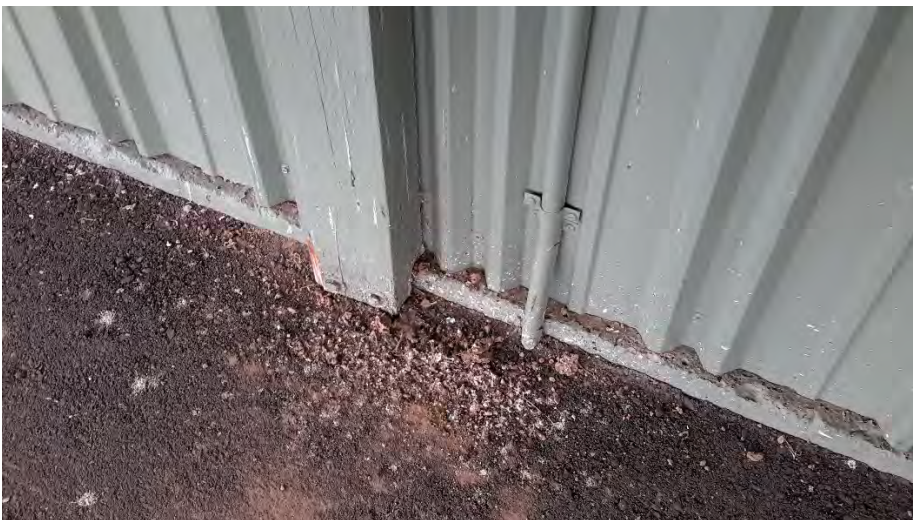
Figure 6 Building 1 - no separation to grade at post base
