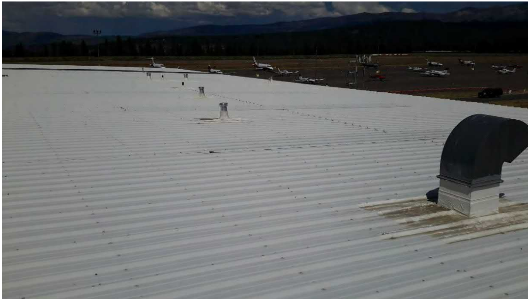
Figure 15 Building 7 - skylight patches
