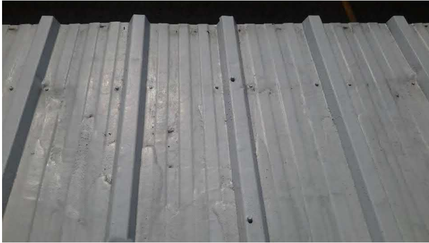
Figure 70 Hangar C - roof was coated over older screws, some missing washers
