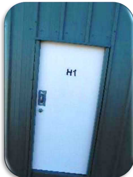
Figure 5-66 shows an example of the condition of the doors on these hangars.
