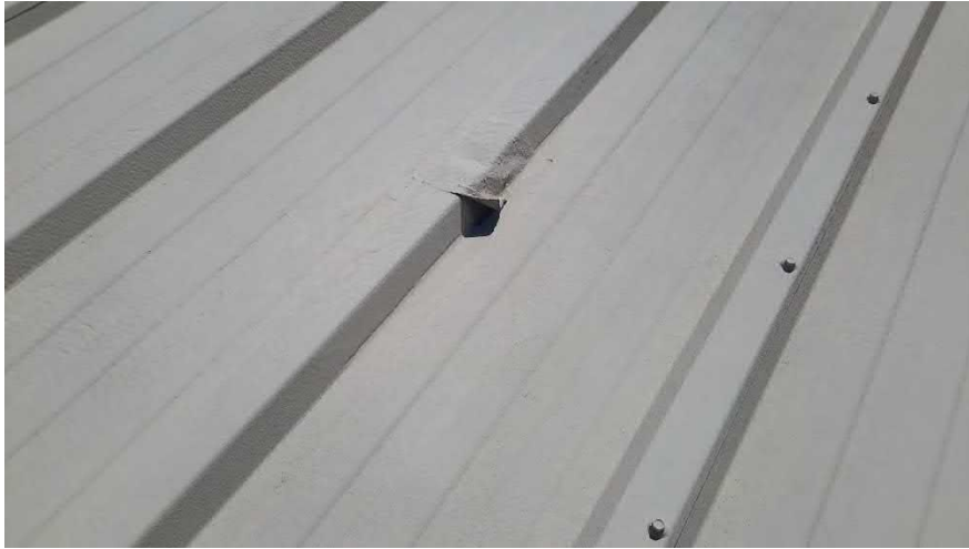
Figure 78 Hangar D - roof coated over older screws, some without washers, fabric patches failing
