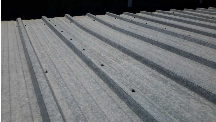
Figure 86 Hangar E - roof panel damage, crimped and kinked from snow and ice damage
