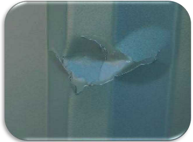
Figure 5-51 shows an example of the impact damage that was observed with the associated coating delaminations
