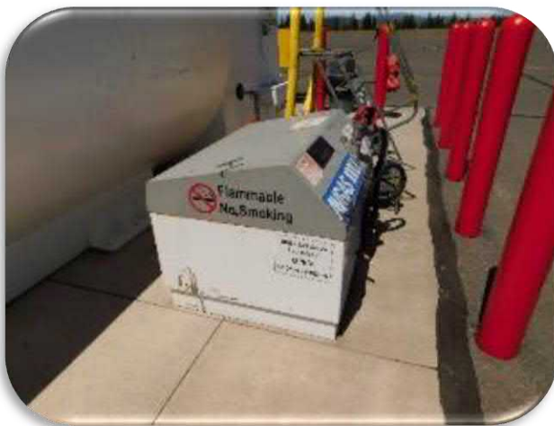
Figure 5-19 shows a general view of the pump enclosure that has edge rusting.
