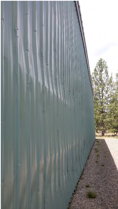
Figure 132 Hangar L - wall panel damage on north side
