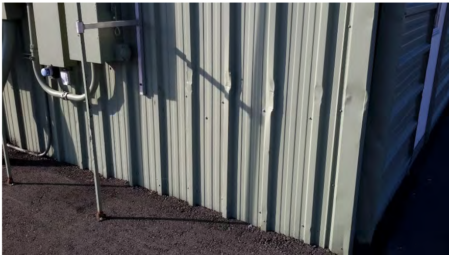
Figure 74 Hangar C - wall panel damage on north end
