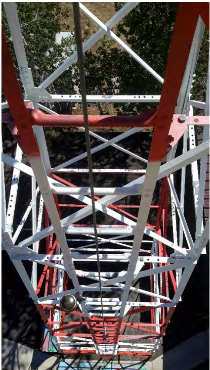
Figure 13 Building 4 - Beacon needs paint
