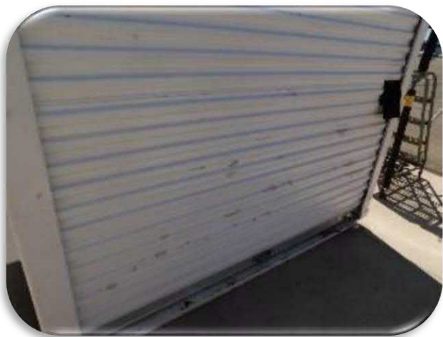
Figure 5-20 shows the delaminations that are present on the roll-up door.
