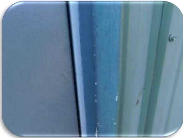
Figure 5-27 shows the faded siding and trim on the maintenance facility. Also note the impact damage on the trim.
