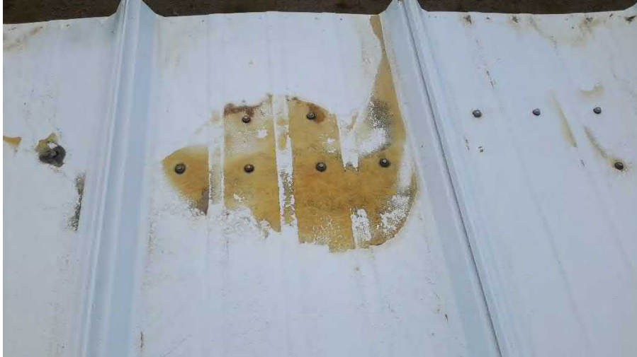
Figure 107 Hangar H - leak patch cracking, low end, east side
