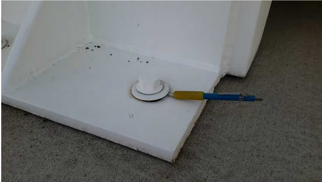
Figure 14 Building 5 - bolts at southwest foot are loose.
