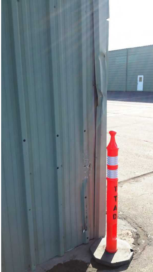
Figure 66 Hangar B - siding damage - south east corner
