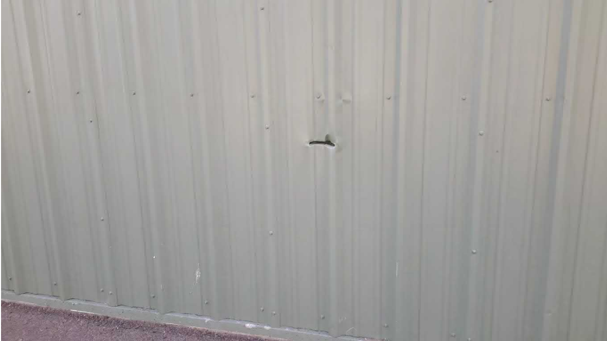
Figure 19 Building 8 - puncture hole - west side
