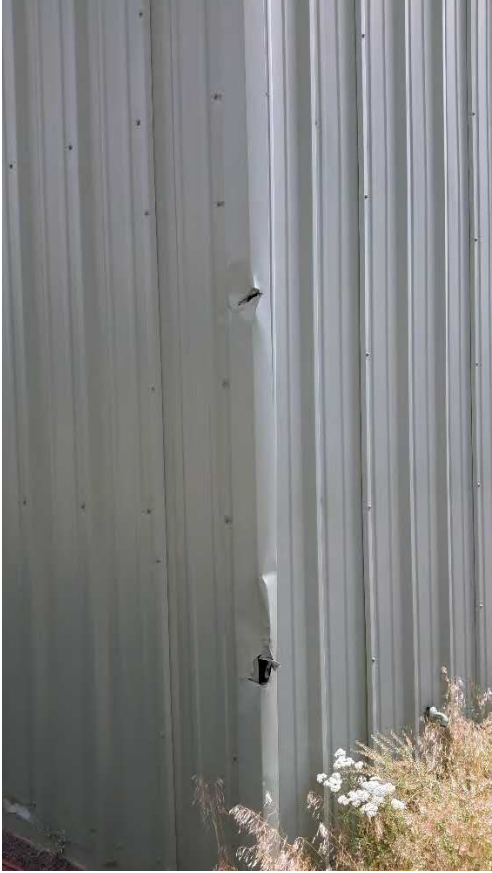
Figure 18 Building 8 - damage at southwest corner
