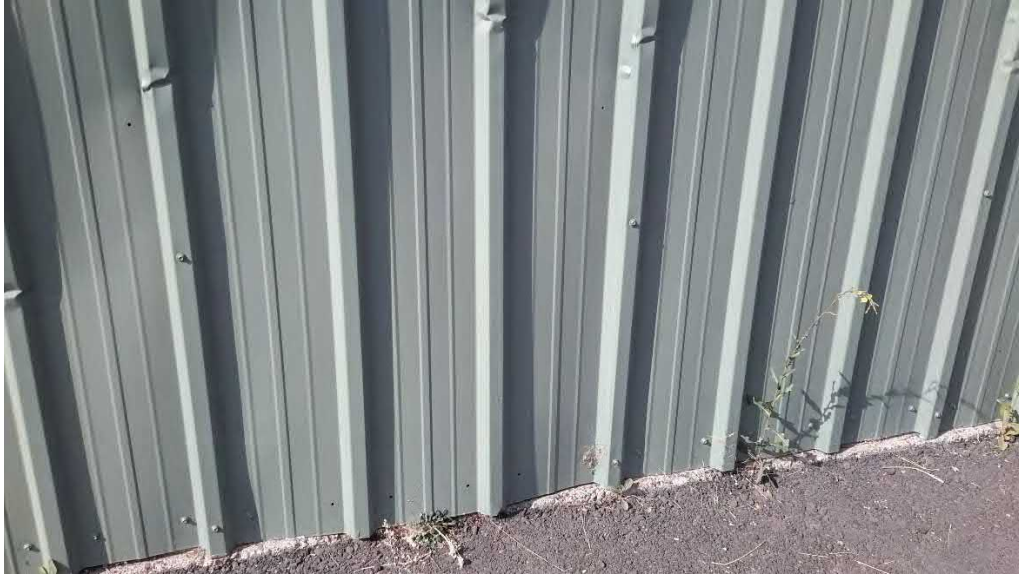
Figure 112 Hangar H - panel fasteners are missing at base of north wall
