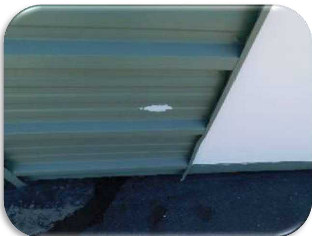
Figure 5-65 shows an example of the infrequent coating delaminations on Hangar B.
