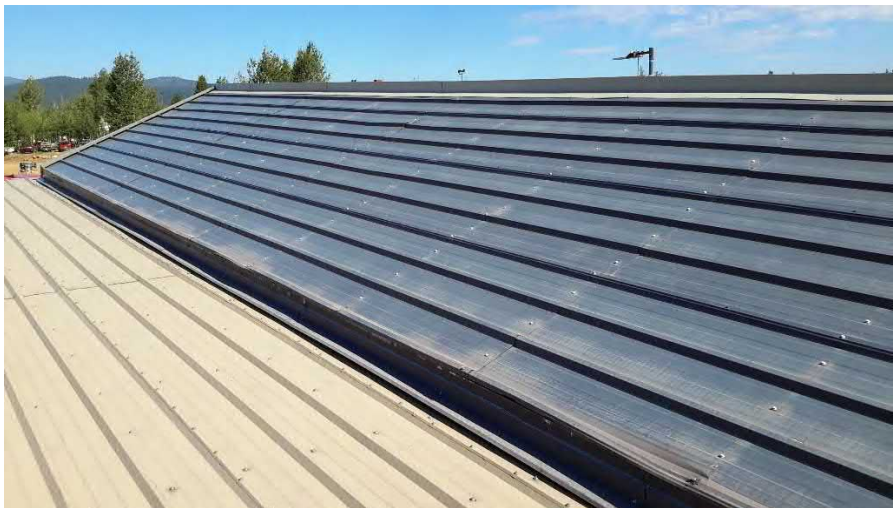
Figure 54 Hangar A - paint coat worn off at over-frame area
