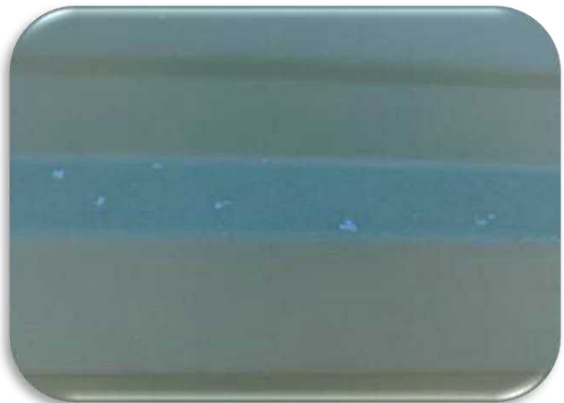
Figure 5-68 shows an example of an areas where the coating has worn away exposing the galvanized substrate.
