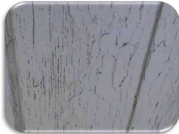
Figure 5-57 shows the typical condition of the wood siding. Note the cracked and lifting paint.
