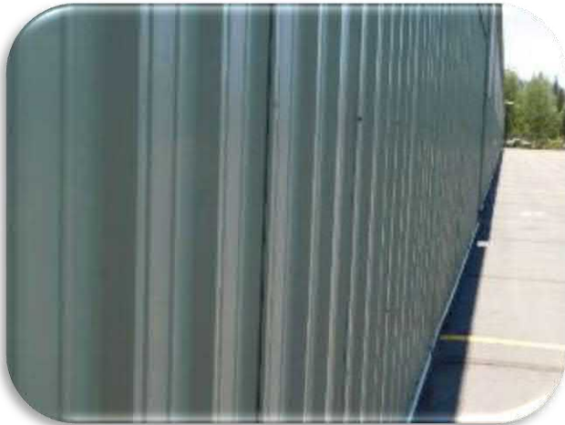
Figure 5-64 shows an example of the condition of the recently painted siding on Hangars A, B and F through H.
