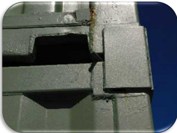
Figure 5-62 shows an example of the rusting that was observed on the Air Traffic Control Tower stairway.
