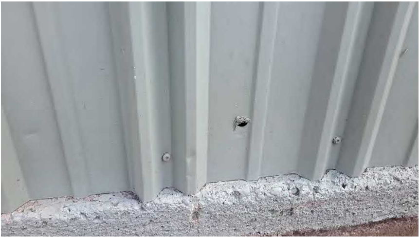
Figure 9 Building 1 - panel damage and loose fasteners
