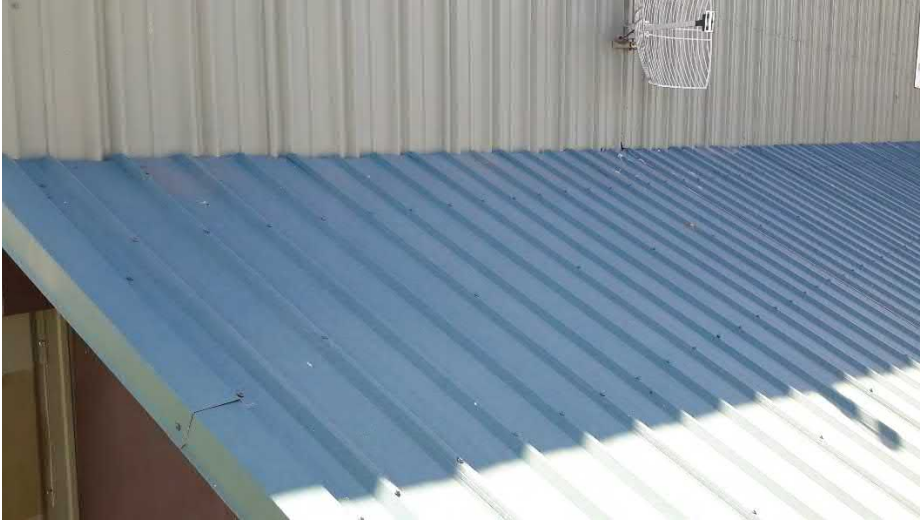
Figure 4 Building 1 - no flashing at top of roof to wall
