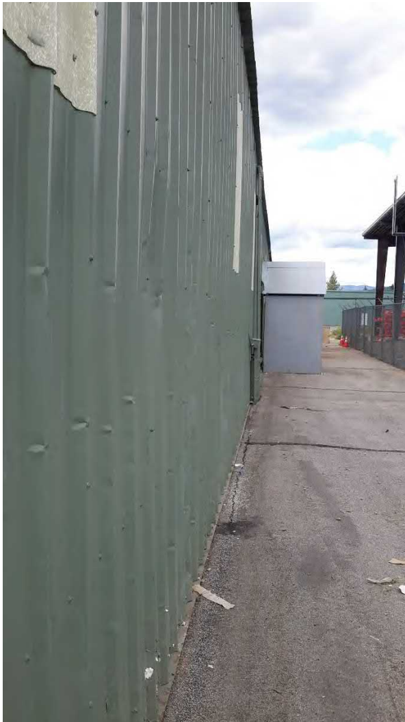
Figure 30 Building 11 - panel damage on north side
