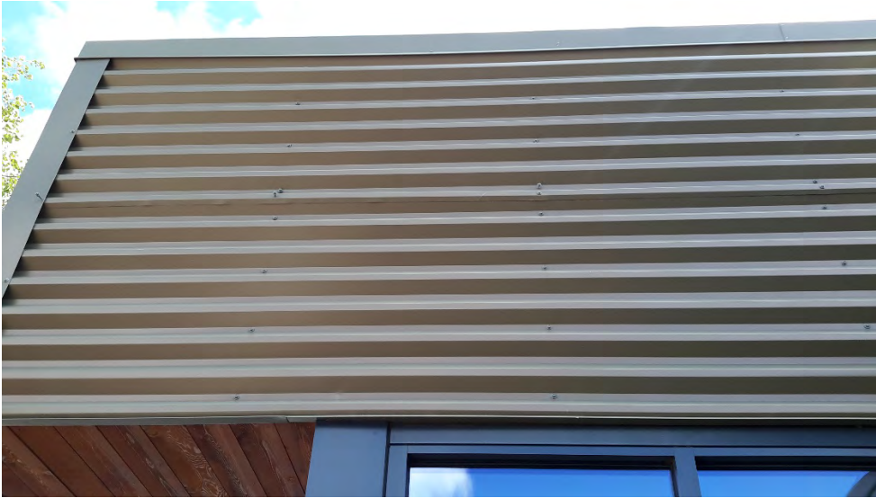
Figure 10 Building 2 - loose screws in fascia - south side at west flat roof
