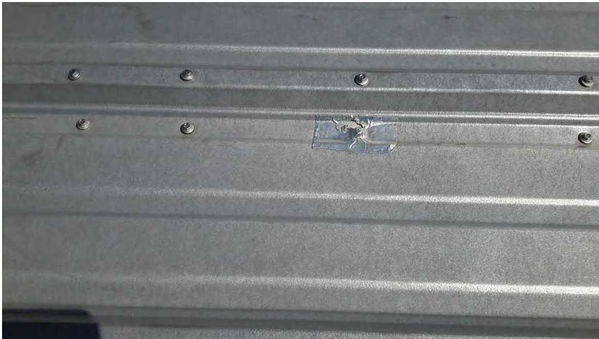
Figure 25 Building 10 - foil-faced adhesive patches damaged
