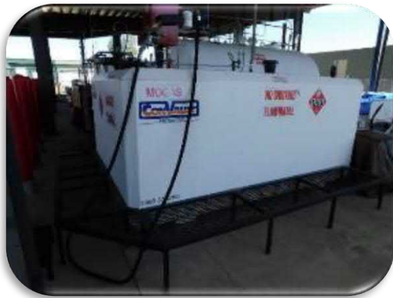
Figure 5-47 shows a general view of the Mogas concrete tank. The coating applied to this tank is free of coating defects.
