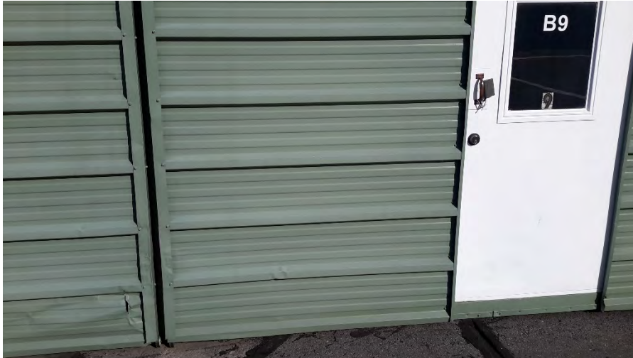
Figure 68 Hangar B - panel damage - east side
