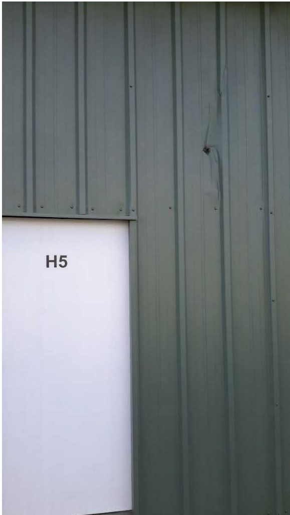
Figure 113 Hangar H - wall panel puncture (H5)
