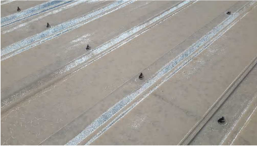
Figure 116 - Hangar J - unconventional fastening system - but no reported leaks
