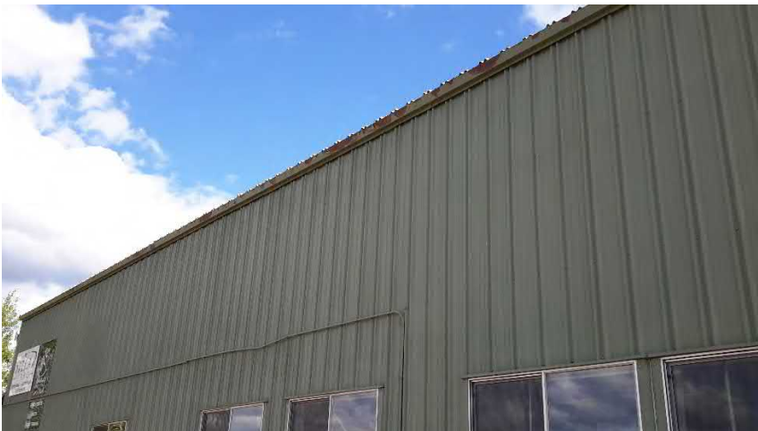
Figure 3 Building 1 - peeling paint on eaves
