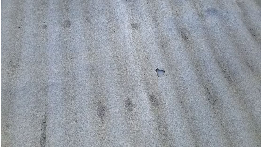
Figure 46 Building 13 - holes in roof, foam below coating damaged
