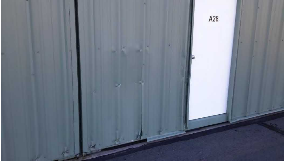
Figure 59 Hangar A - wall panel damage along west side
