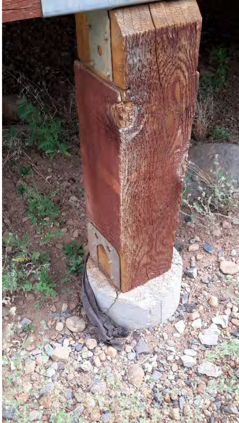
Figure 24 Building 9 - south west deck - pier cracked and failing
