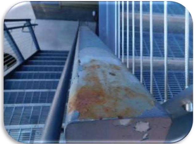
Figure 5-11 shows an example of the extensive coating delaminations and rusting that is occurring on the stairway handrails.
