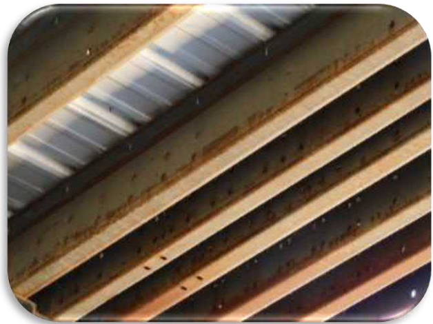
Figure 5-35 shows a general view of the roof rafters that support the roof structure. Note the edge and pinpoint rusting on the rafters.
