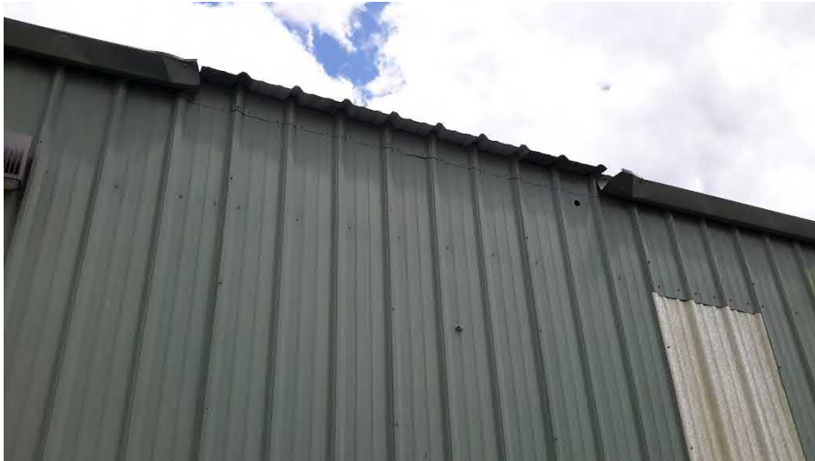
Figure 33 Building 11 - gutter damage on south side
