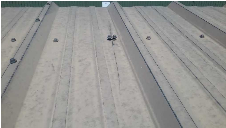
Figure 94 Hangar F - loose screws evident on roof
