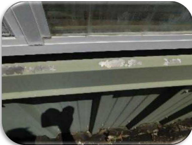
Figure 5-71 shows the delamination on the galvanized windowsill.
