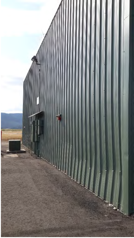
Figure 110 Hangar H - wall panel damage on north end
