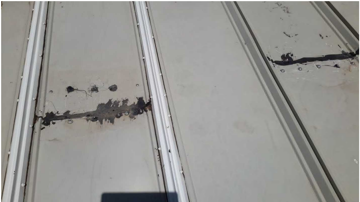
Figure 136 Hangar M - numerous attempts to patch leaks
