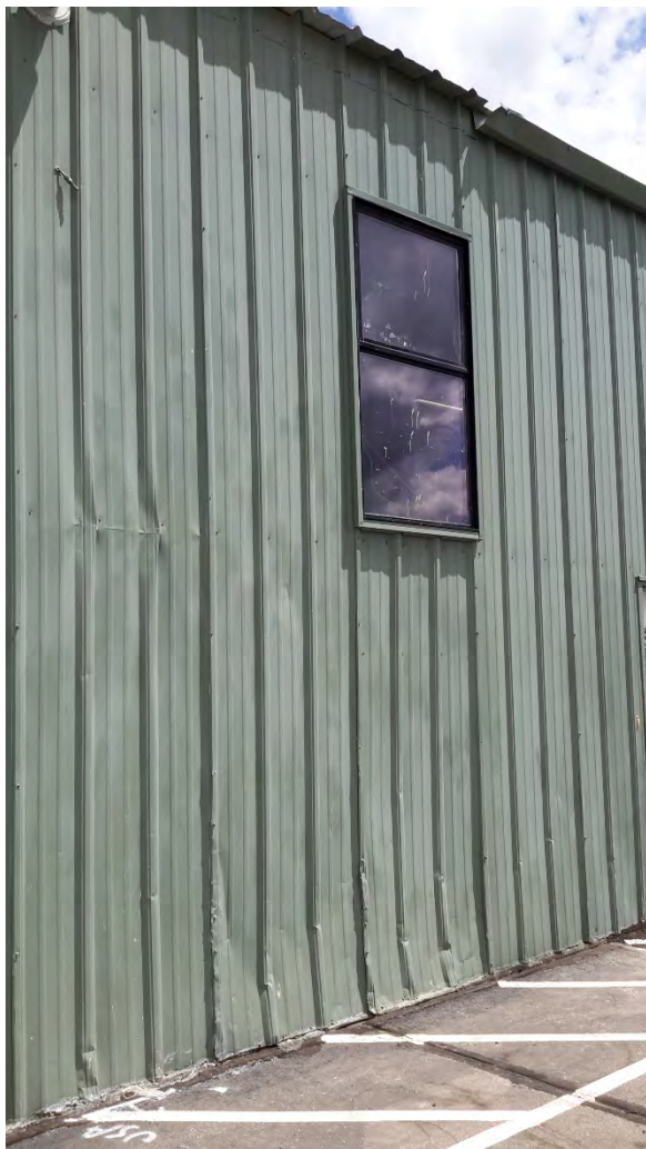
Figure 34 Building 11 - wall panel damage on south side from snow, ice and/or vehicles
