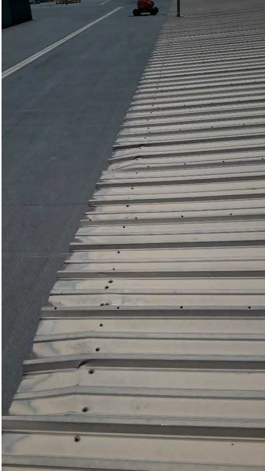
Figure 125 Hangar K - damage to low (east) side roof panels from snow and ice.
