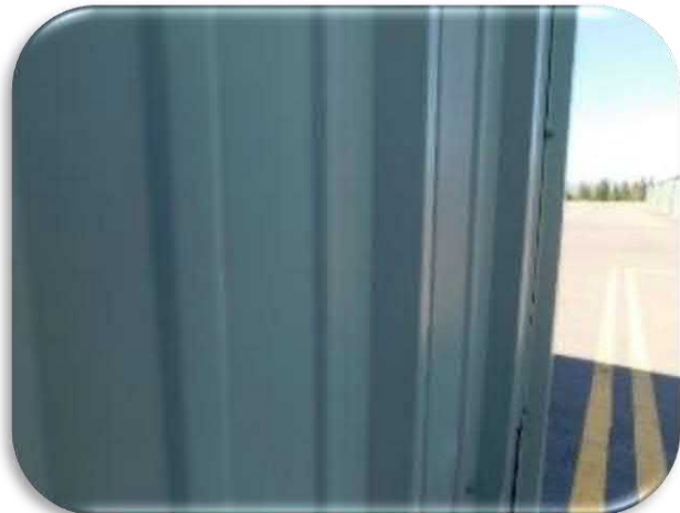
Figure 5-30 shows the appearance of the siding. Note that it is glossy and free of coating defects.
