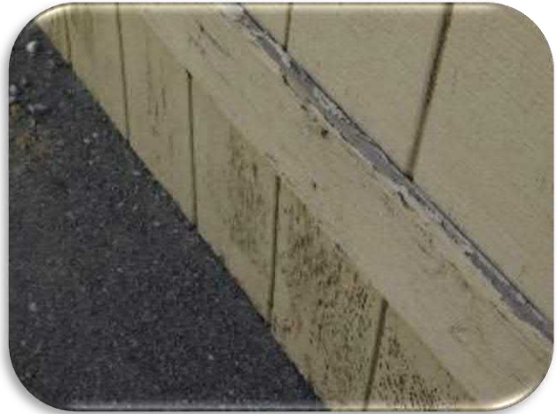
Figure 5-32 shows the condition of the T-111 siding. Note the coating delaminations and cracked wood.
