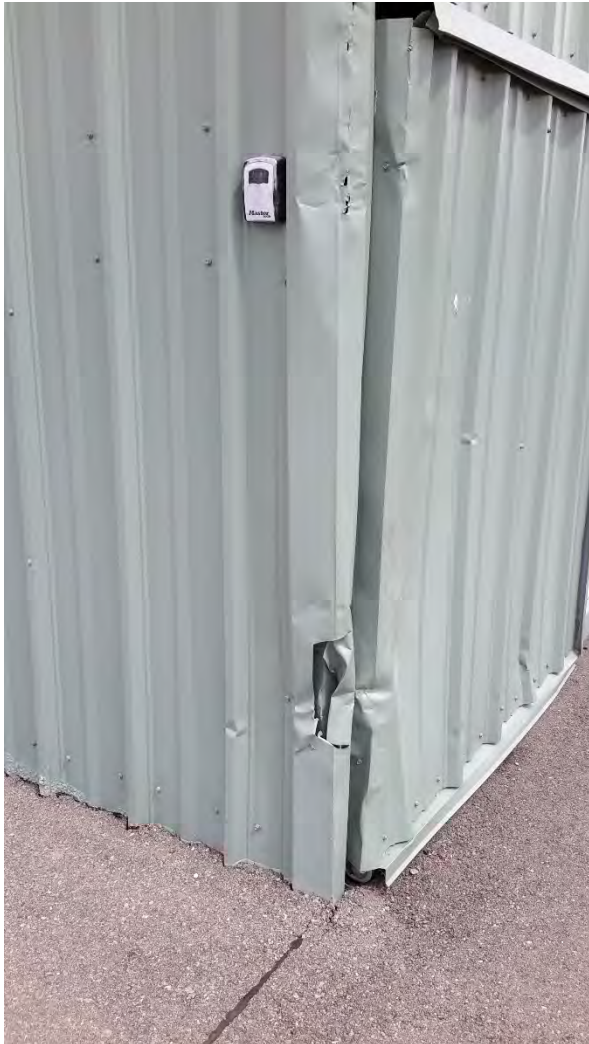
Figure 128 Hangar K - wall panel damage on south east corner
