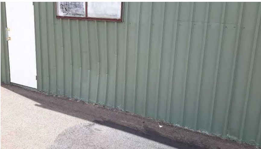
Figure 118 Hangar J - wall panel damage north end
