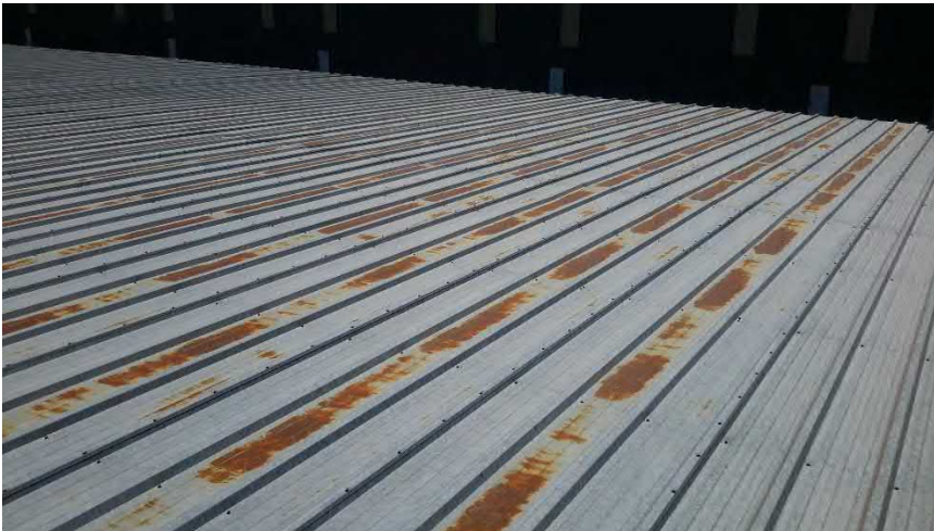
Figure 84 Hangar E - large areas of rust on roof panels
