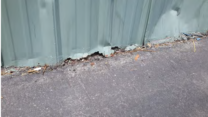
Figure 37 Building 11 - panel damage / corrosion on east side
