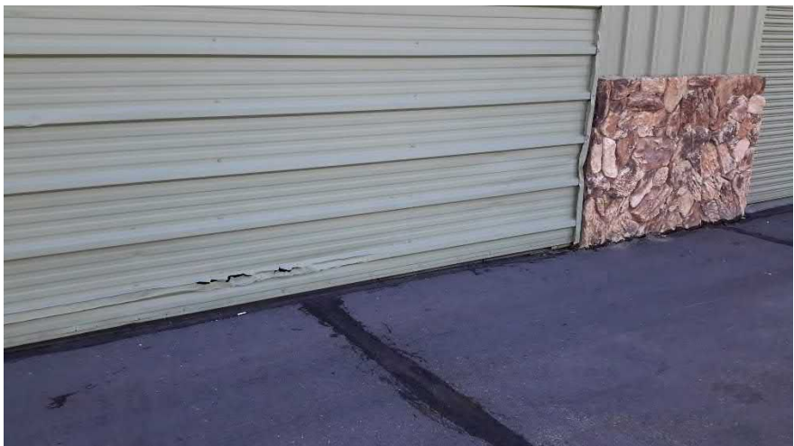
Figure 75 Hangar C - wall panel damage - west side (C24)
