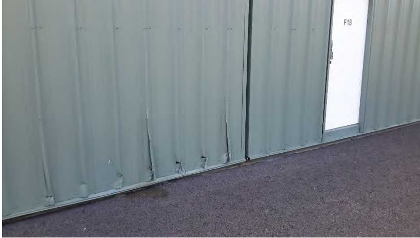
Figure 100 Hangar F - door panel damage (F16)
