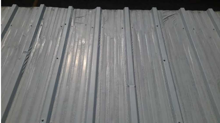
Figure 73 Hangar C - roof coating delaminating from roof panels
