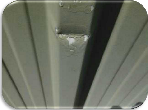
Figure 5-70 shows a delamination at an impact point.
