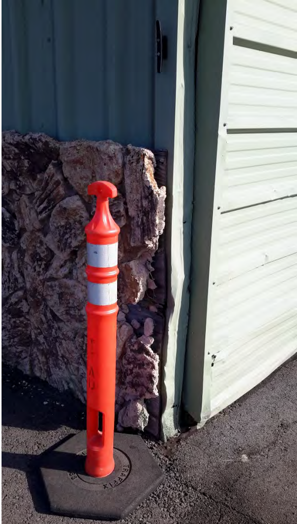
Figure 76 Hangar C - wall panel damage - south east corner
