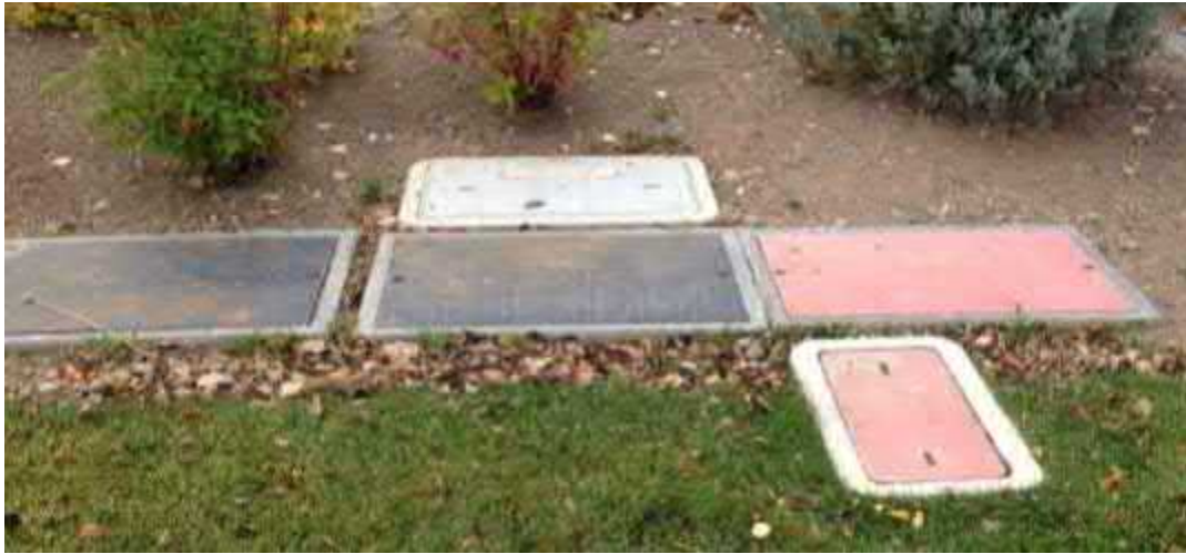
Figure 9-8. Communication and Power Pull-Boxes
