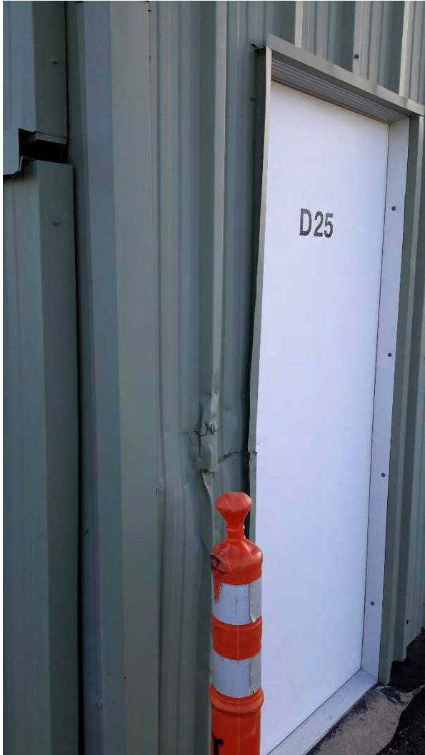
Figure 81 Hangar D - wall panel damage at south west corner
