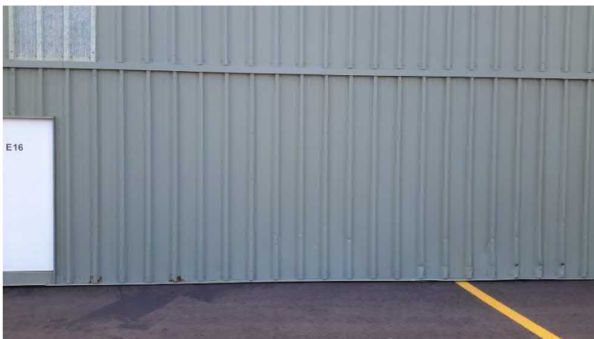
Figure 88 Hangar E - base of door (E16) has damage and rust evident
