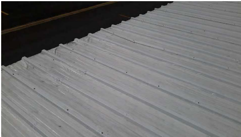
Figure 71 Hangar C - roof panels damaged from snow and ice
