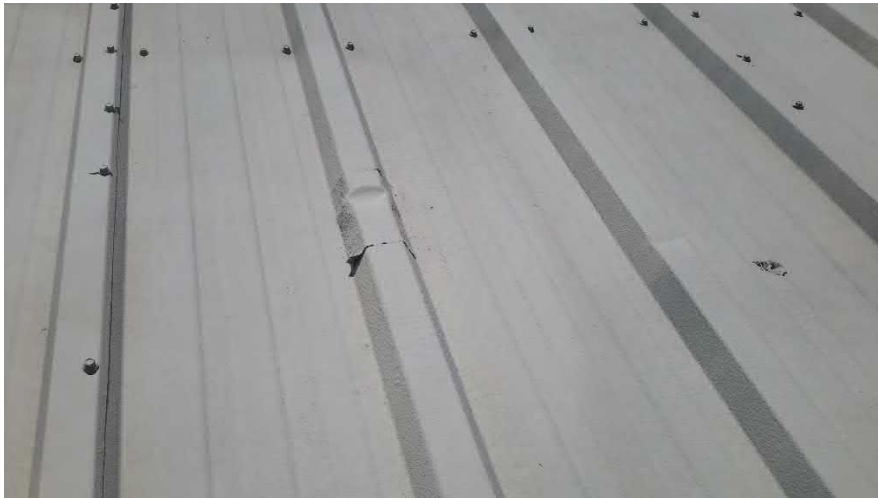
Figure 79 Hangar D - fabric patches failing, roof panels kinked / crimped
