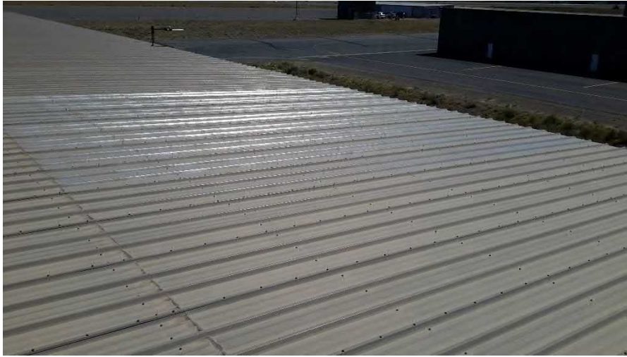
Figure 93 Hangar F - roof panel paint coat badly worn
