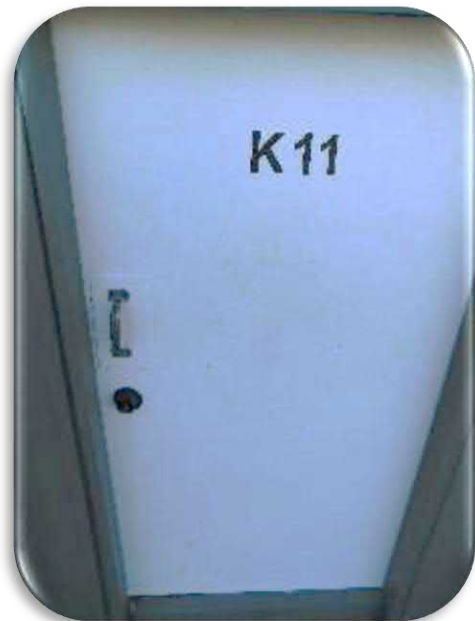
Figure 5-78 shows the typical condition of the doors on these hangars.
