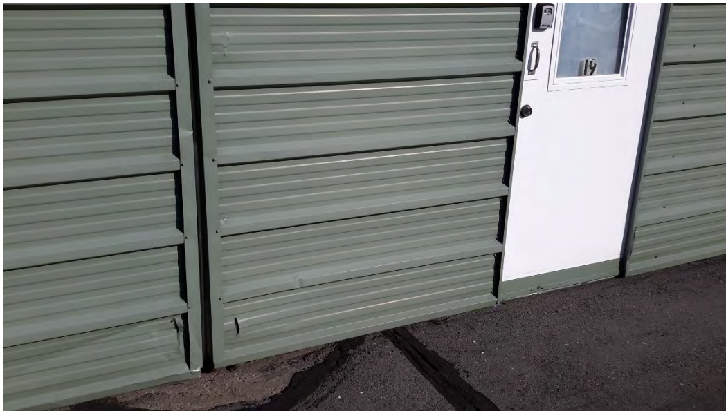
Figure 67 Hangar B - Panel damage - east side
