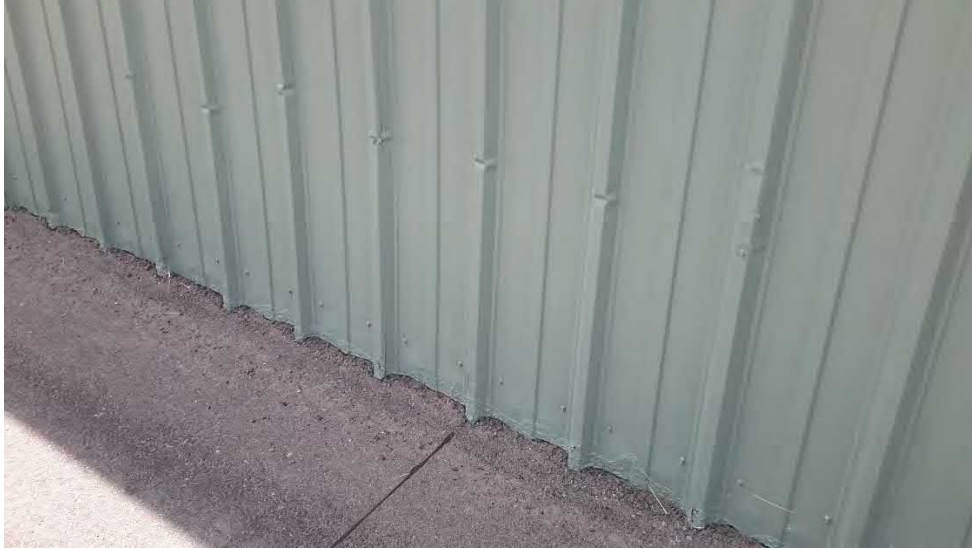
Figure 127 Hangar K - wall panel damage on north end
