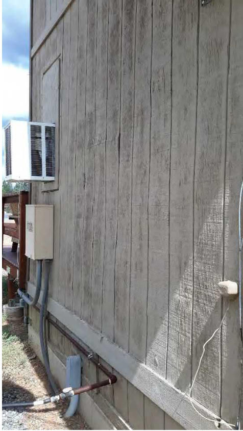
Figure 22 Building 9 - south side wall siding buckled
