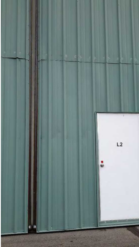
Figure 135 Hangar L - rust at door track / column
