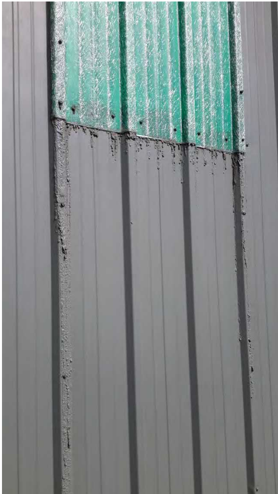
Figure 115 Hangar H - sealant to translucent panels, east side, poor installation
