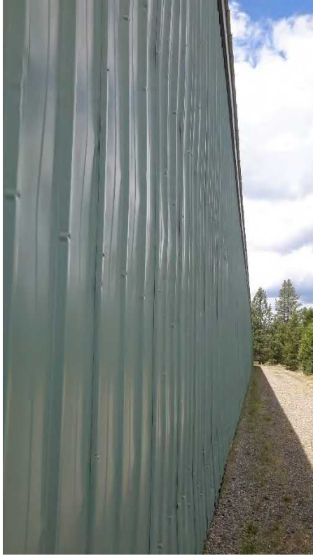
Figure 131 Hangar L - wall panel damage on north side
