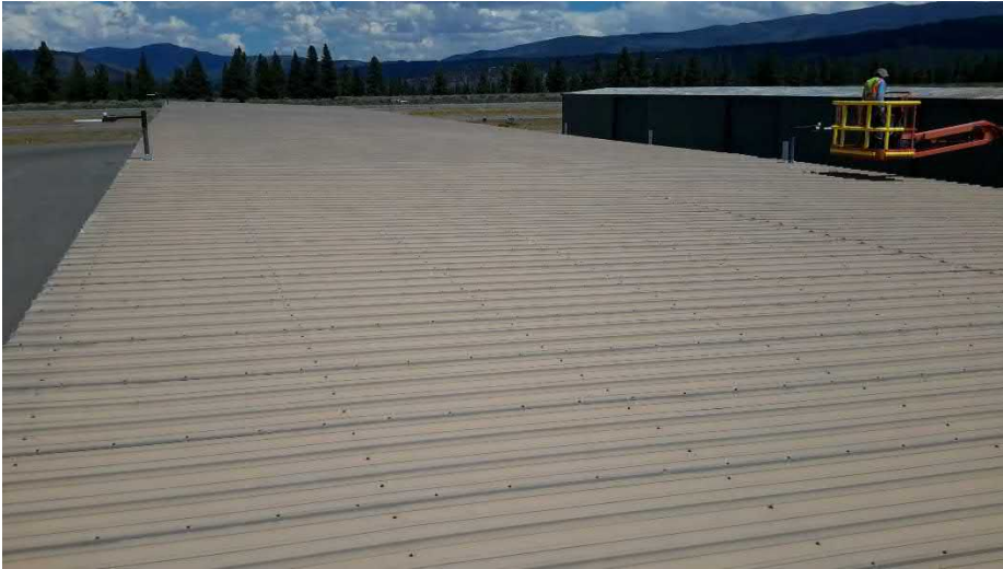
Figure 121 Hangar K - paint coat is badly worn
