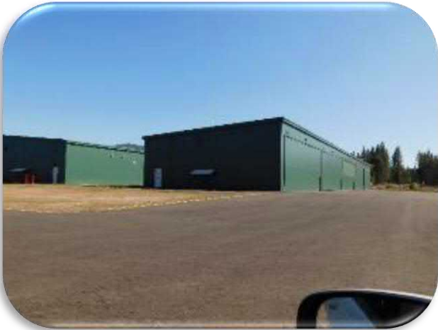
Figure 5-79 shows a general view of Hangars N and P--Not the glossy appearance of the recently applied coating system.
