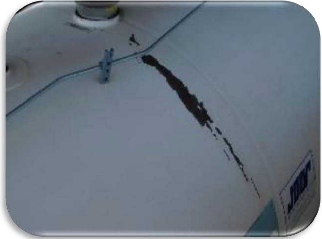
Figure 5-40 shows the coating degradation that was observed directly beneath the fill ports.
