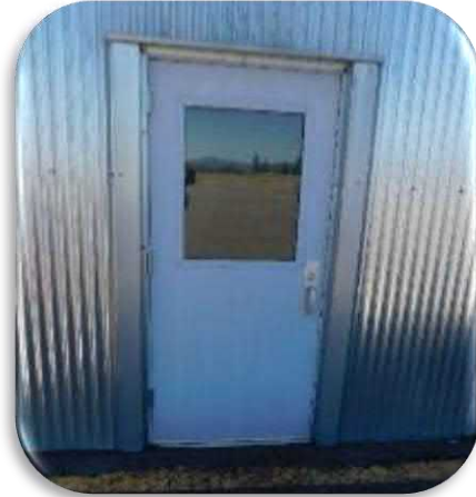
Figure 5-4 shows the general condition of the doors that have not been recently painted.
