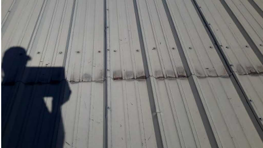
Figure 53 Hangar A - corrosion at lap seam in middle of roof
