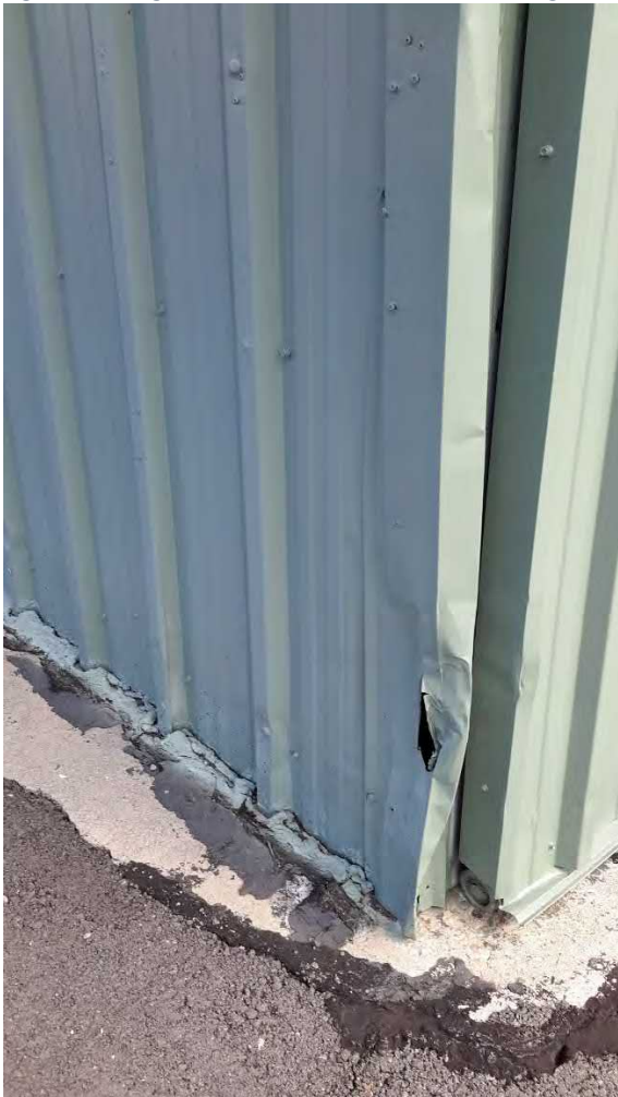
Figure 92 Hangar E - wall panel damage at south east corner
