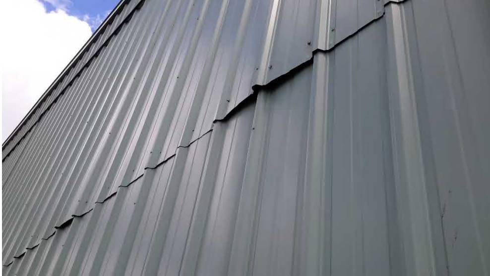
Figure 133 Hangar L - door panel loose and missing fasteners
