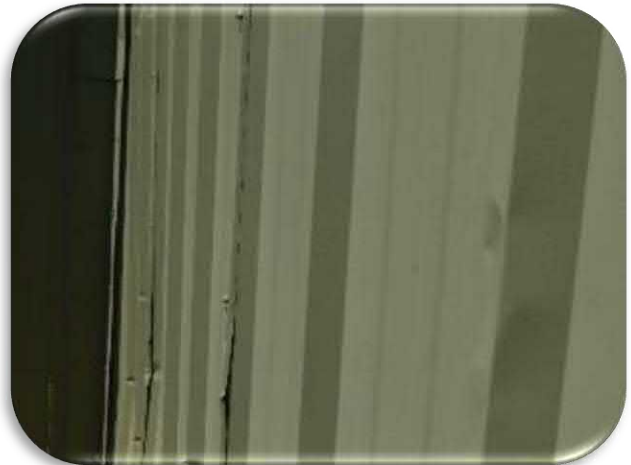
Figure 5-55 shows an example of the impact damage that was present on the hangar surfaces.
