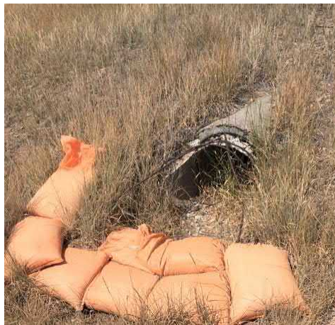
Figure 8-1 Exposed Rebar on Culvert 118
