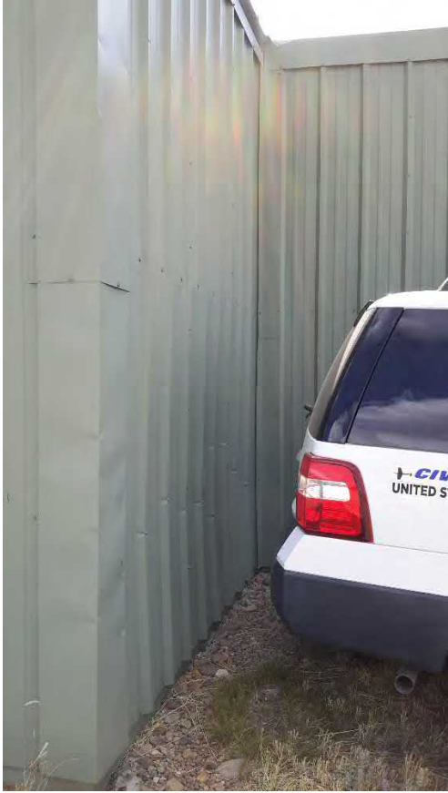
Figure 44 Building 12 - wall panel damage from snow and ice
