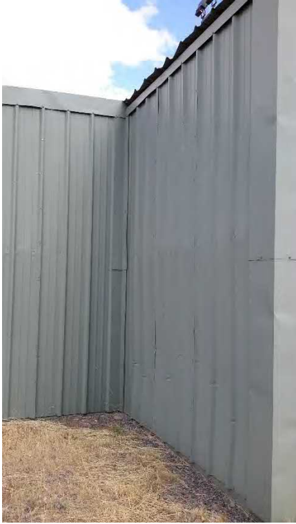
Figure 42 Building 12 - wall panel damage from snow and ice
