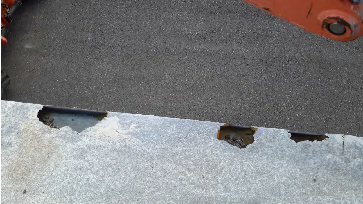
Figure 45 Building 13 - numerous holes in roof
