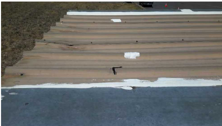
Figure 39 Building 12 - roof is in poor condition
