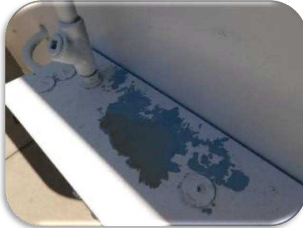
Figure 5-21 shows the delaminations on the electrical box.
