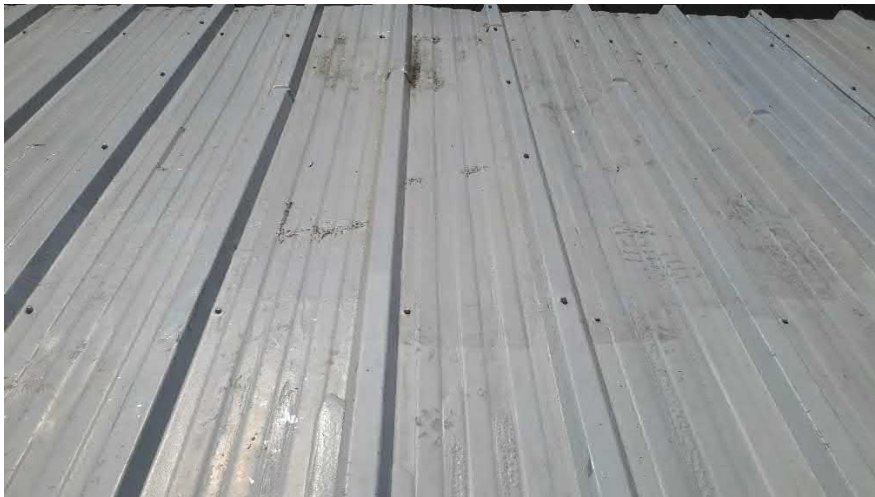
Figure 63 Hangar B - roof panels crimped / kinked from snow and ice damage
