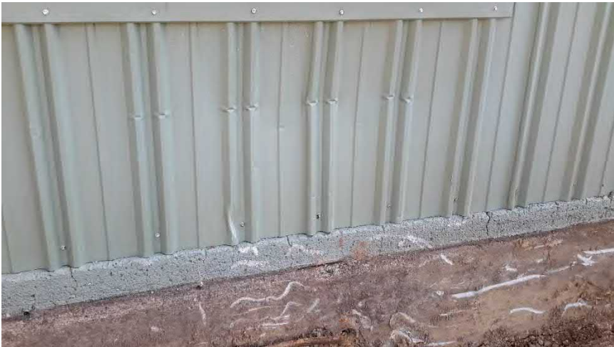
Figure 8 Building 1 - panel damage from snow
