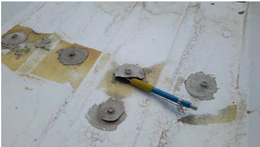
Figure 109 Hangar H - leak patch on low end (east side) failing, screws loose
