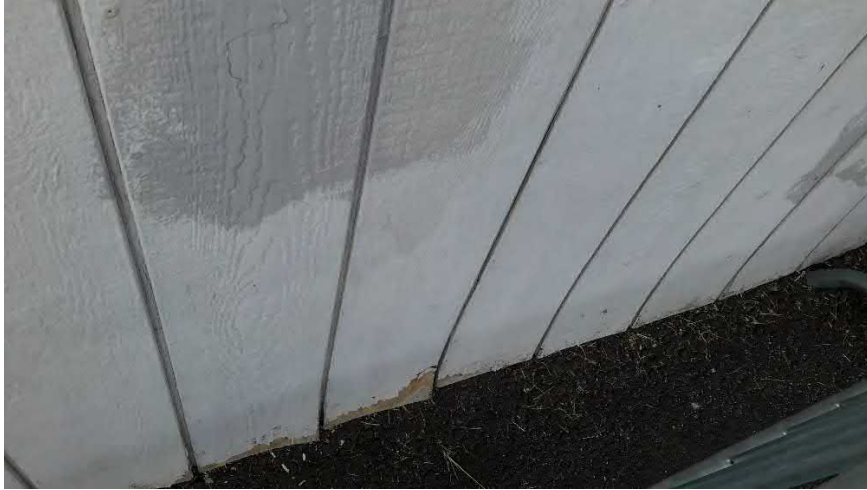
Figure 50 Building 13 - north side of building, siding is buckled, wood siding extends down to grade level
