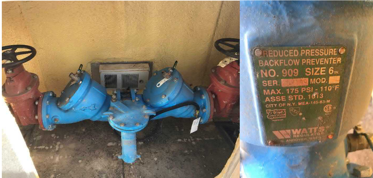
Figure 9-2. 6" Watts Reduced Pressure Backflow Preventer in hot box
