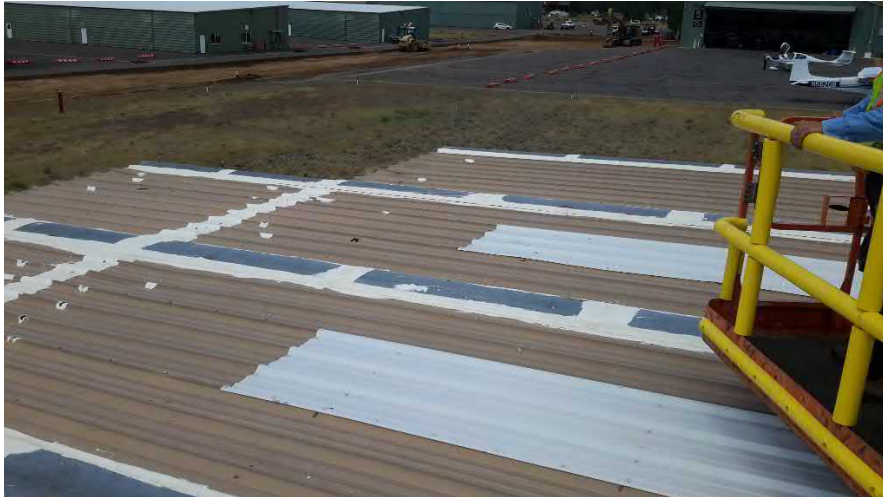
Figure 38 Building 12 - roof patchwork
