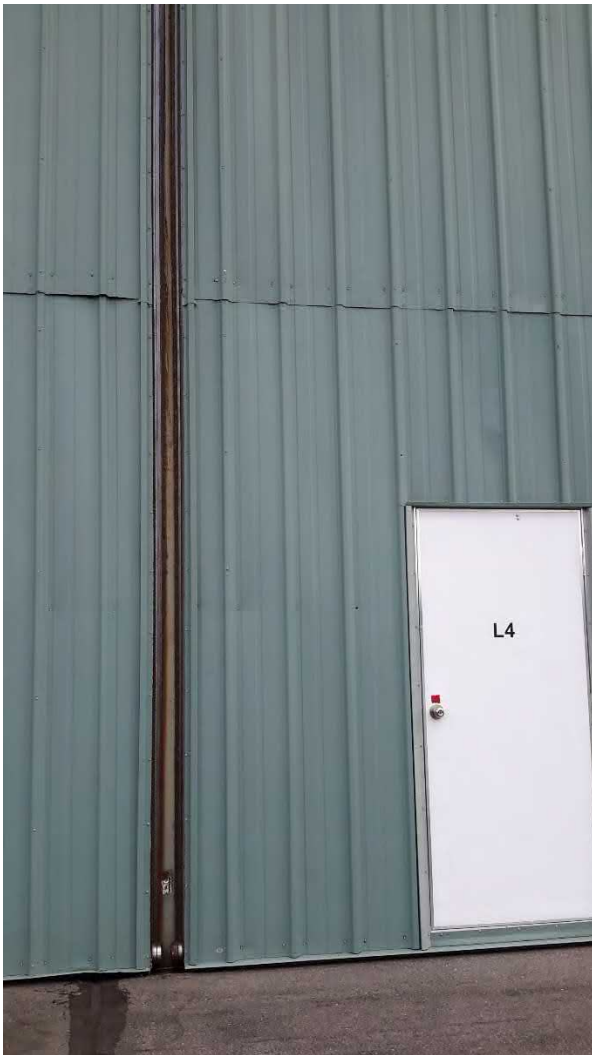
Figure 134 Hangar L - rust at door track / columns
