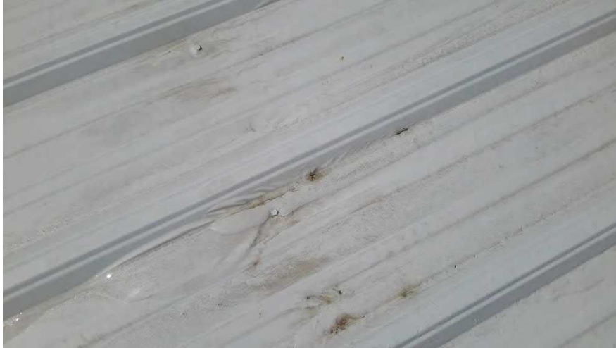
Figure 29 Building 11 - pockets of water under roof coating
