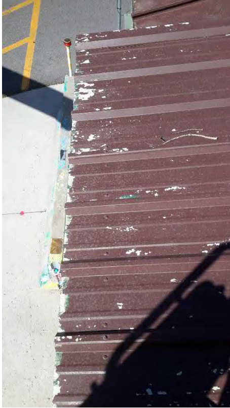
Figure 12 Building 3 - paint missing / corrosion at eaves
