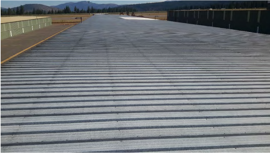
Figure 83 Hangar E - paint coat on roof non-existent
