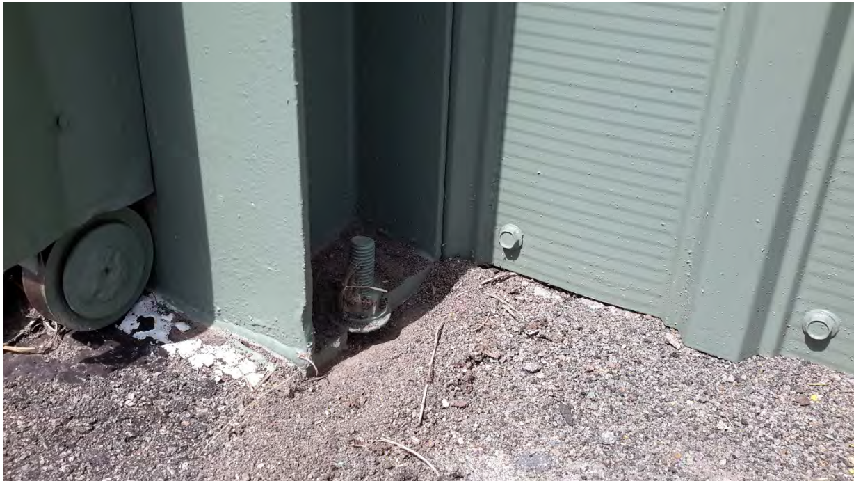
Figure 120 Hangar J - column anchor bolt mis-placed
