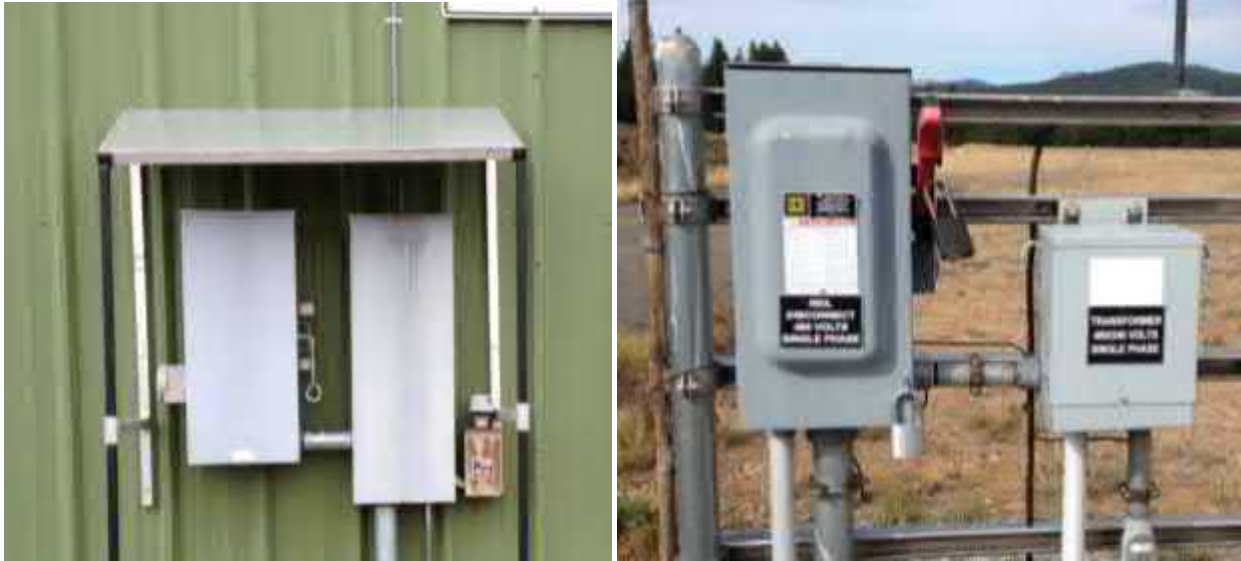
Figure 9-6 and Figure 9-7. Power Distribution Panels
