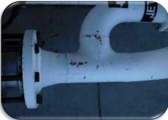
Figure 5-45 shows the typical degree of impact damage and rust on the pumping station surfaces.
