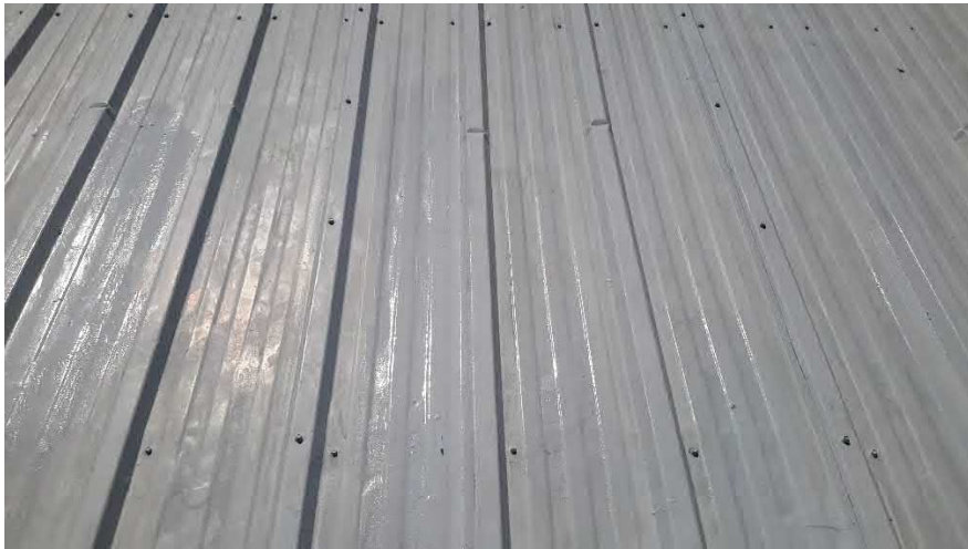
Figure 62 Hangar B - roof panels crimped / kinked from snow and ice damage
