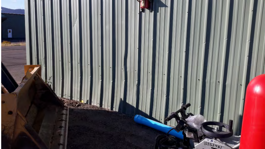
Figure 56 Hangar A - north end wall panels damaged from snow and ice
