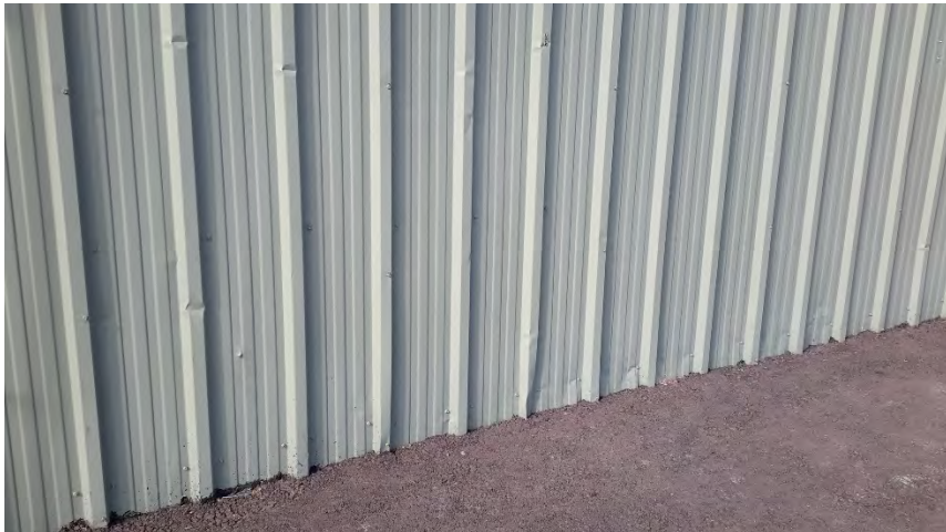
Figure 87 Hangar E - wall panel damage on north end from snow and ice
