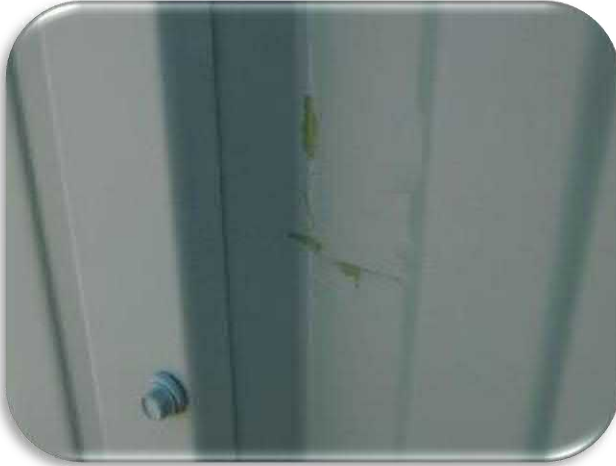
Figure 5-69 shows one example of the blistered that were observed on the siding.
