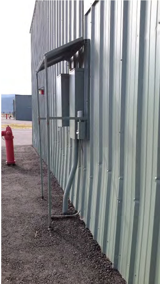
Figure 98 Hangar F - wall panel damage on north end from snow and ice
