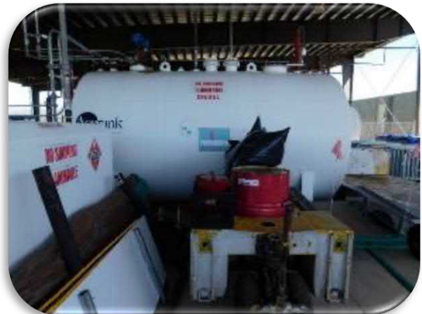
Figure 5-46 shows a general view of the diesel fuel storage tank. The coatings applied to this tank are in good condition.
