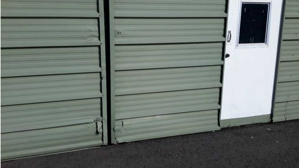
Figure 77 Hangar C - wall panel damage - east side (C13)
