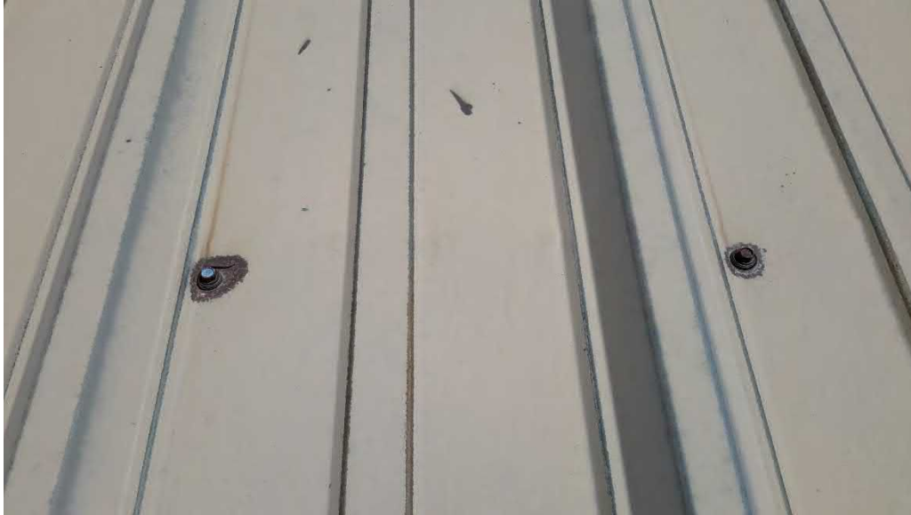
Figure 123 Hangar K - neoprene washers disintegrating and rust at screws
