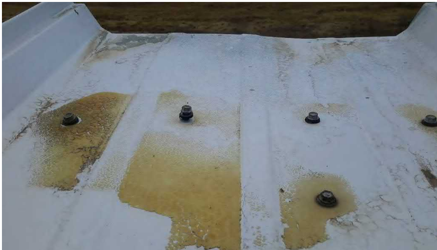
Figure 108 Hangar H - low end (east side) screws loose and leak patch failing
