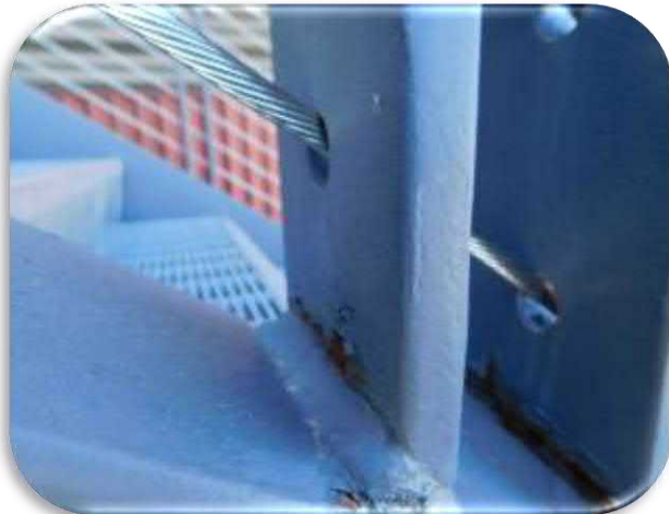
Figure 5-8 shows rusting at the base of the railing posts where water puddles.
