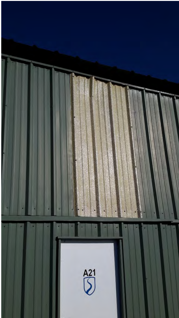
Figure 60 Hangar A - translucent panel damage - east side
