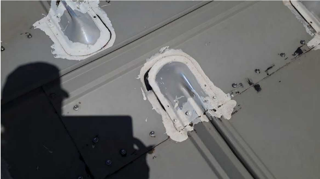
Figure 138 Hangar M - gaskets and sealant loose at ridge line
