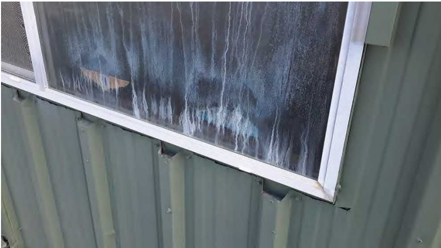
Figure 90 Hangar E - window trim on south wall missing
