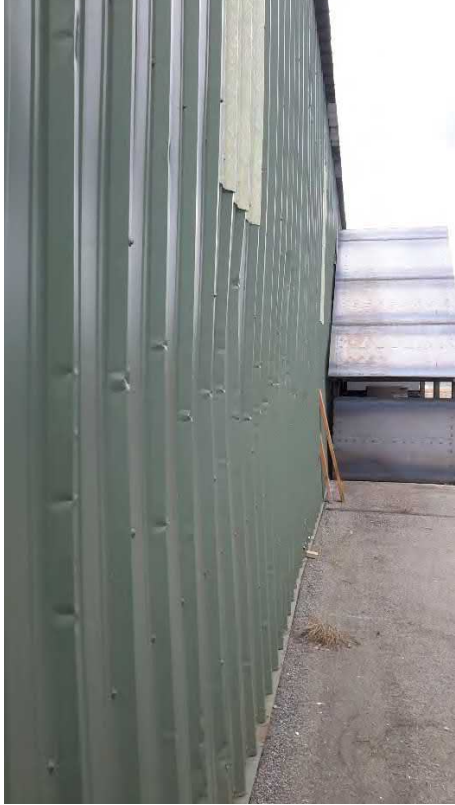
Figure 31 Building 11 - panel damage, north side
