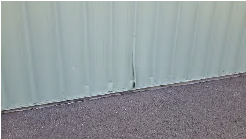
Figure 101 Hangar F - door panel damage (F18)
