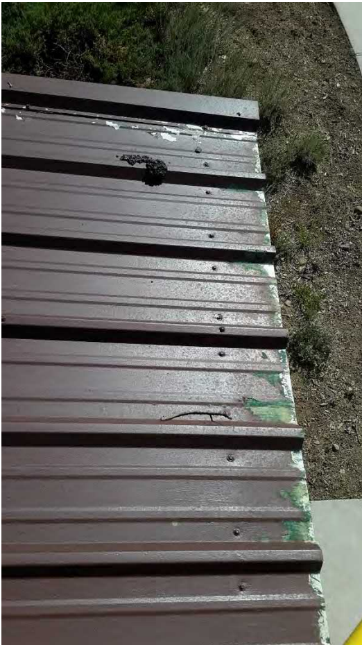
Figure 11 Building 3 - paint missing / corrosion at eave
