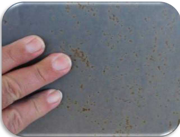
Figure 5-37 shows an example of the pinpoint rusting that was present on the structural steel.
