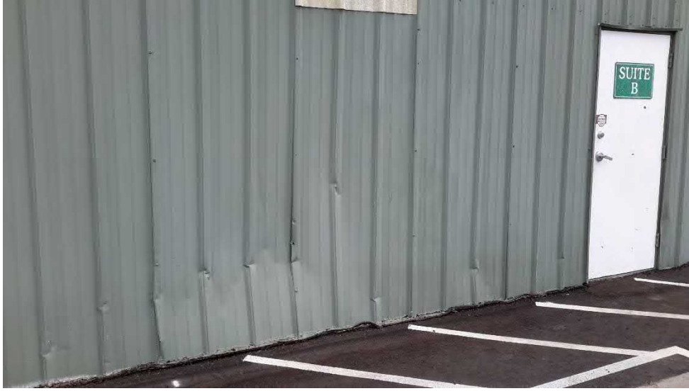
Figure 35 Building 11 - wall panel damage on south side from snow, ice and/or vehicles
