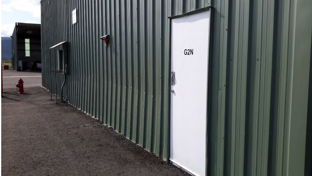
Figure 103 Hangar G - wall panel damage on north end from snow and ice
