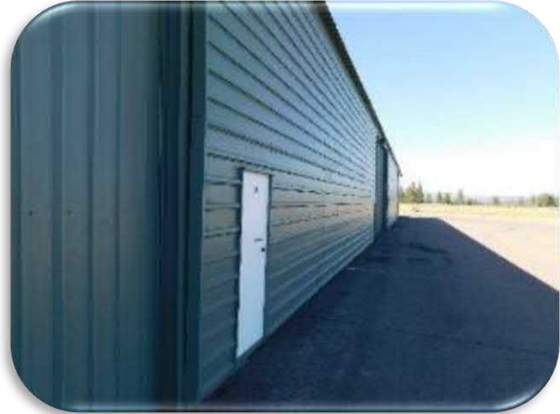
Figure 5-77 shows a general view of the coating condition on Hangars J through M. Note the freshly painted glossy appearance.
