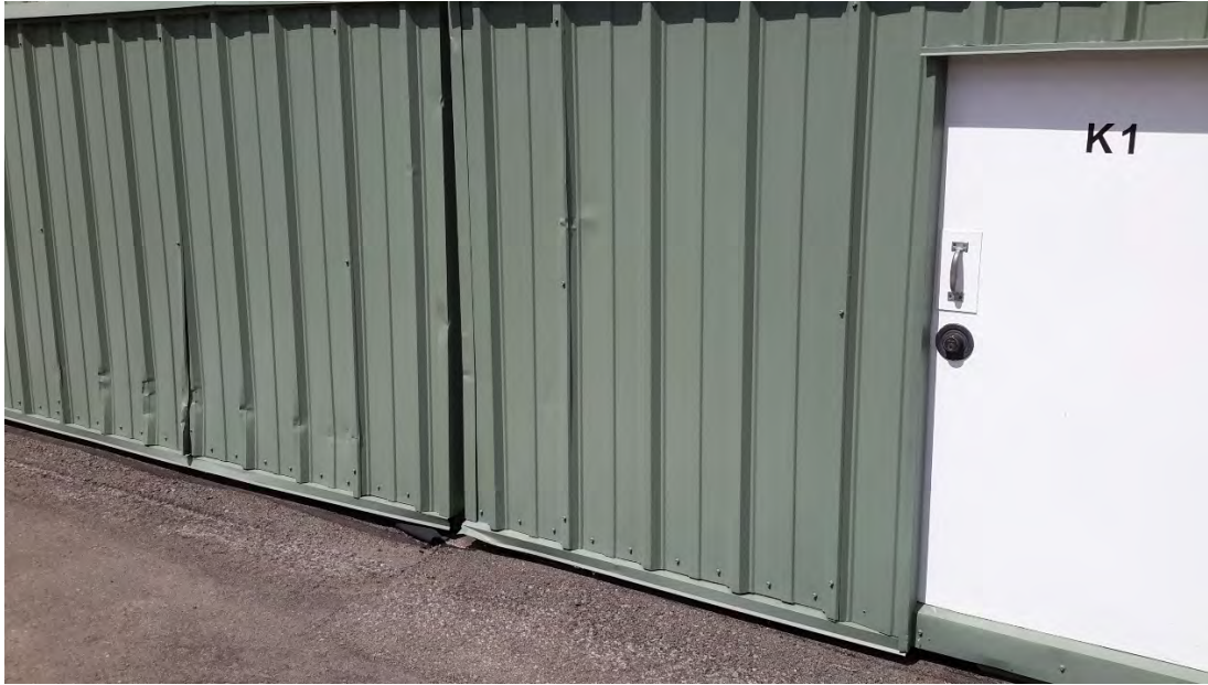
Figure 129 Hangar K - door panel damage (K3)
