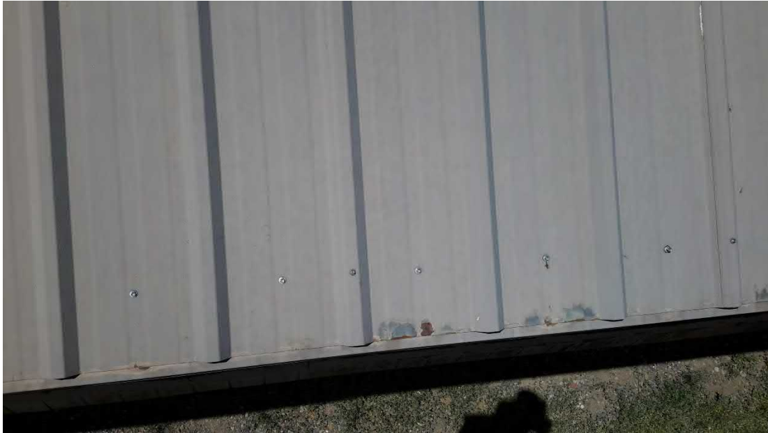
Figure 20 Building 9 - paint peel and corrosion on east eave
