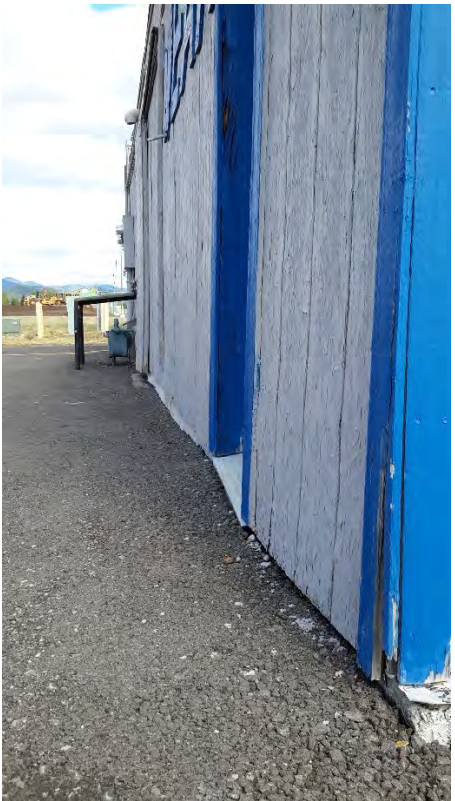
Figure 49 Building 13 - siding corner trim damaged, south east corner
