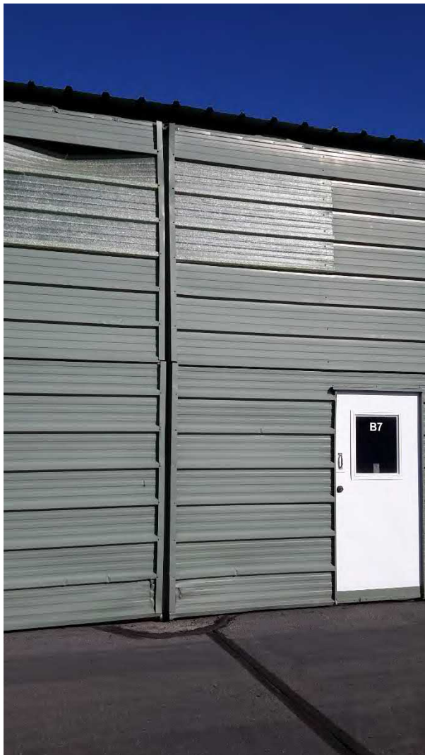
Figure 69 Hangar B - translucent panel damage - east side
