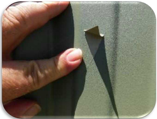
Figure 5-74 shows an example of an adhesion test indicating poor coating adhesion.
