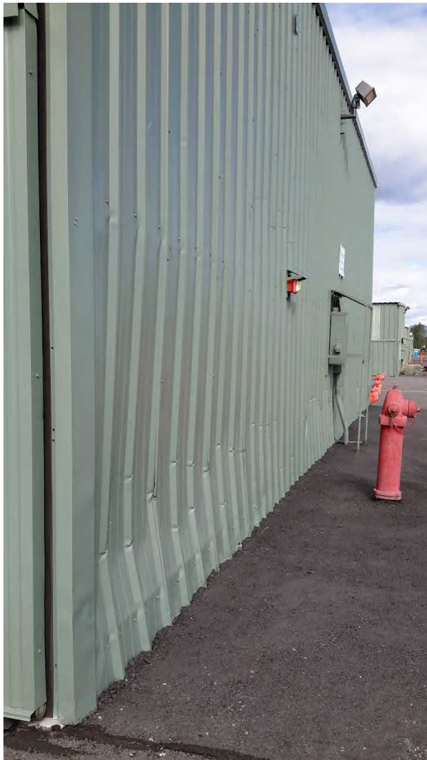
Figure 97 Hangar F - wall panel damage on north end from snow and ice
