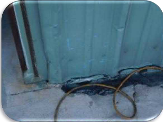
Figure 5-3 shows an example of the impact damage at the base of the siding and the associated coating delaminations
