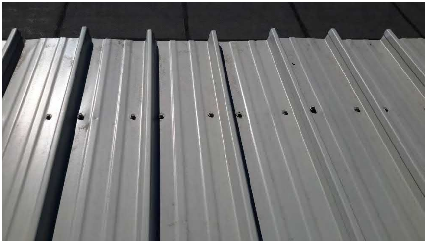
Figure 52 Hangar A - loose screws need to be tightened and/or replaced
