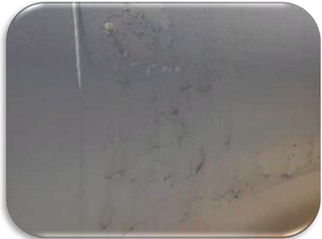
Figure 5-18 shows the delaminations that are present on both sides of the tank.
