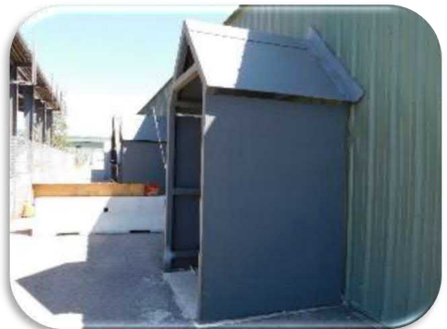
Figure 5-53 shows a general view of the steel entrance ways. The edges of these structures are rusted.
