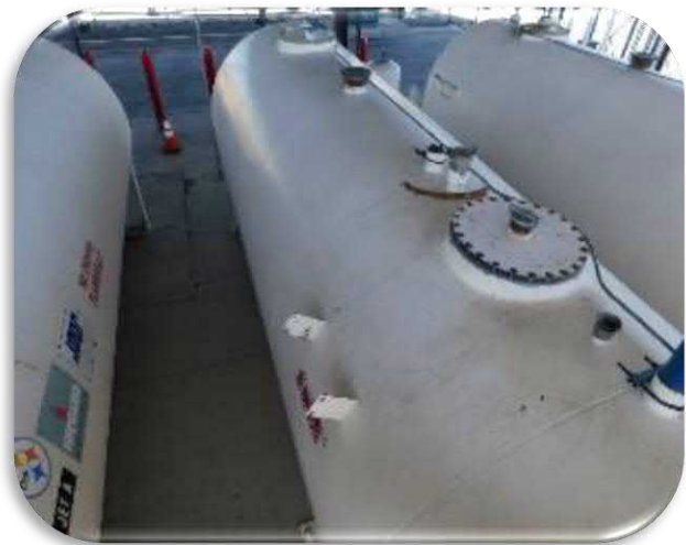
Figure 5-36 shows an example of the typical condition of the seismic rods that are covered in rust.
