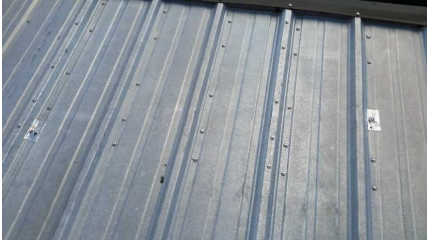
Figure 26 Building 10 - foil-faced adhesive patches damaged.
