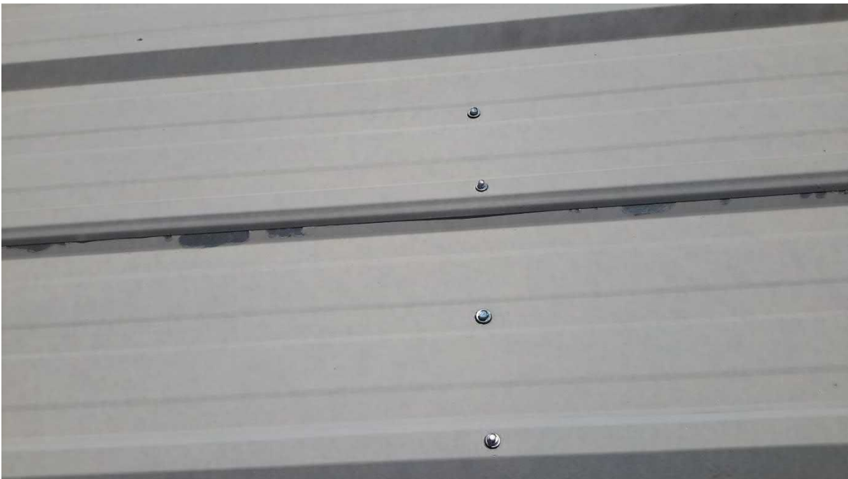
Figure 17 Building 8 - paint flaking on roof panels
