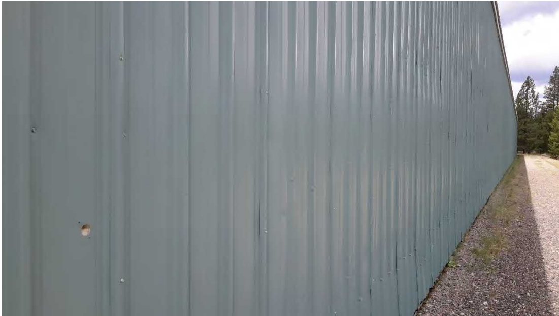
Figure 130 Hangar L - wall panel damage on north side
