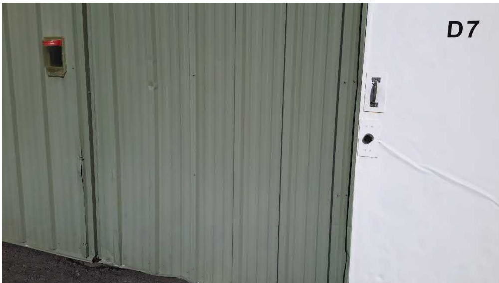
Figure 82 Hangar D - door panel damage (D9)
