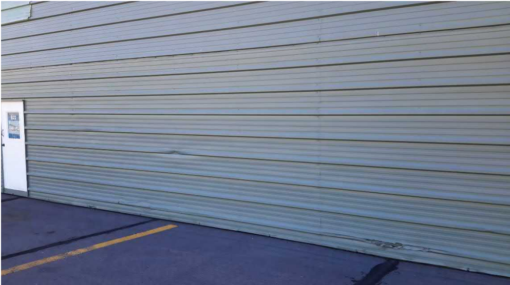
Figure 65 Hangar B - wall panel damage on west side (B22)
