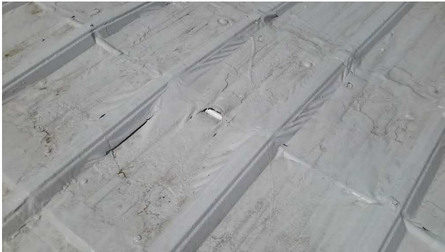
Figure 27 Building 11 - roof coating damaged and delaminating
