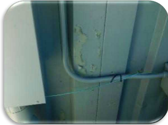
Figure 5-15 shows the small area of coating delaminations on the south side of the building.
