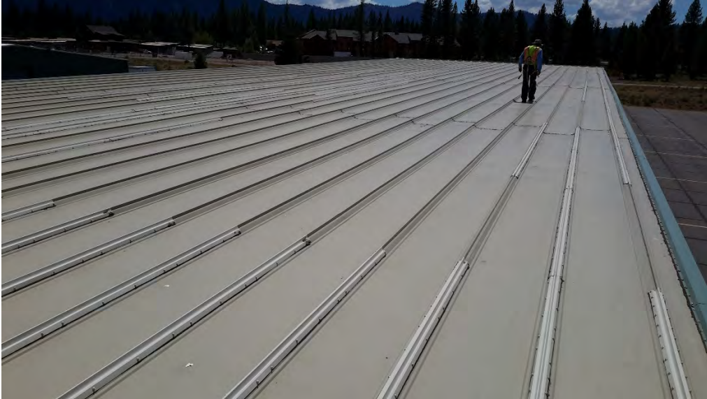
Figure 137 Hangar M - retrofit pieces installed at standing seams to try and fix leaks
