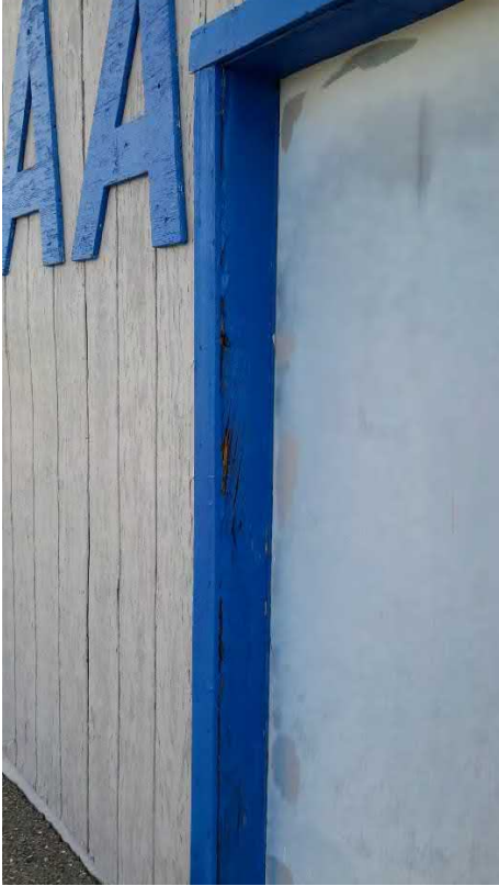
Figure 48 Building 13 - trim, door jamb, paint damaged
