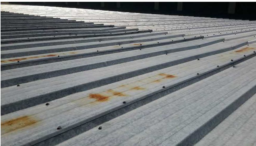
Figure 85 Hangar E - roof panel damage, crimped and kinked from snow and ice damage
