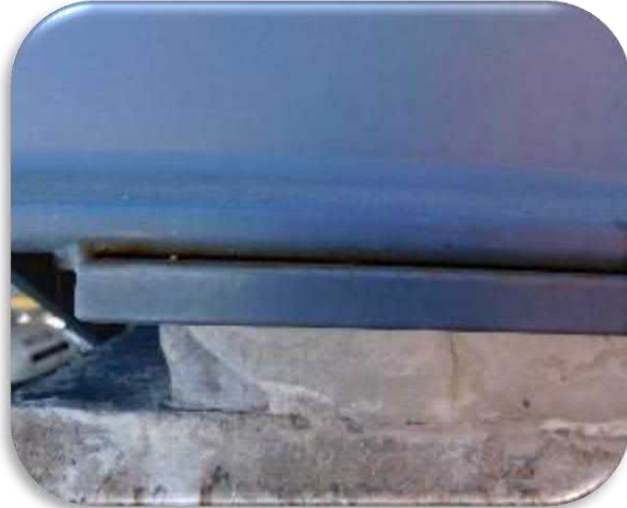
Figure 5-6 shows the rust and rust staining that is present on the stairway structure.
