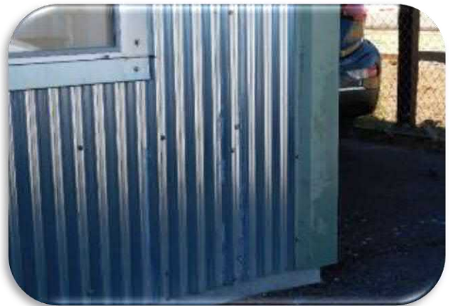
Figure 5-2 shows the unpainted galvanized steel siding. Also note the coating delaminations on the trim at the right of the photo.
