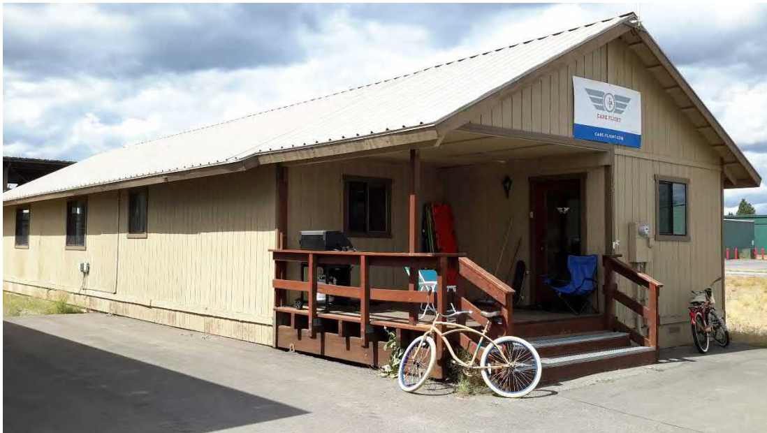
Figure 21 Building 9 - skirt board needs protective paint
