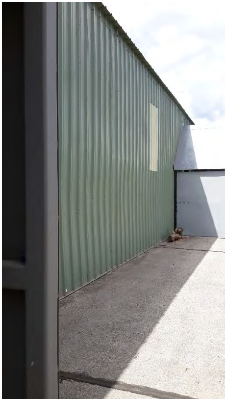
Figure 32 Building 11 - panel damage, north side
