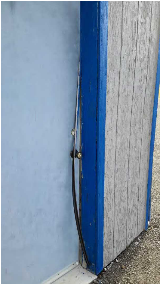
Figure 47 Building 13 - flaking paint, door weather-stripping, door trim damaged
