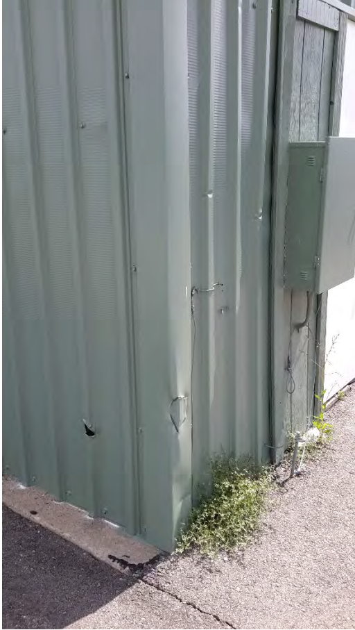
Figure 119 Hangar J - wall panel damage on south west corner
