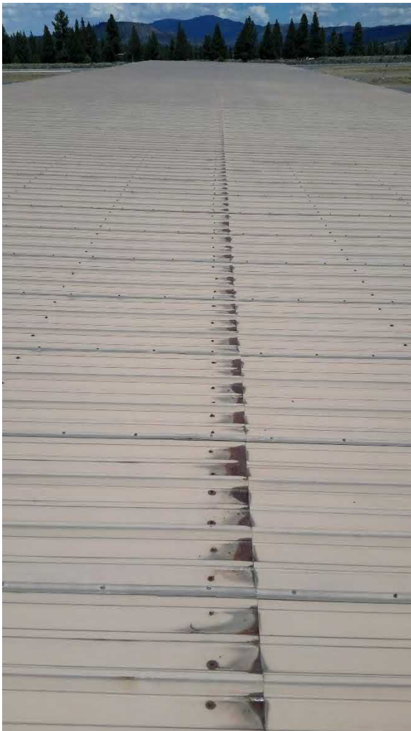
Figure 122 Hangar K - areas of rust and corrosion on roof
