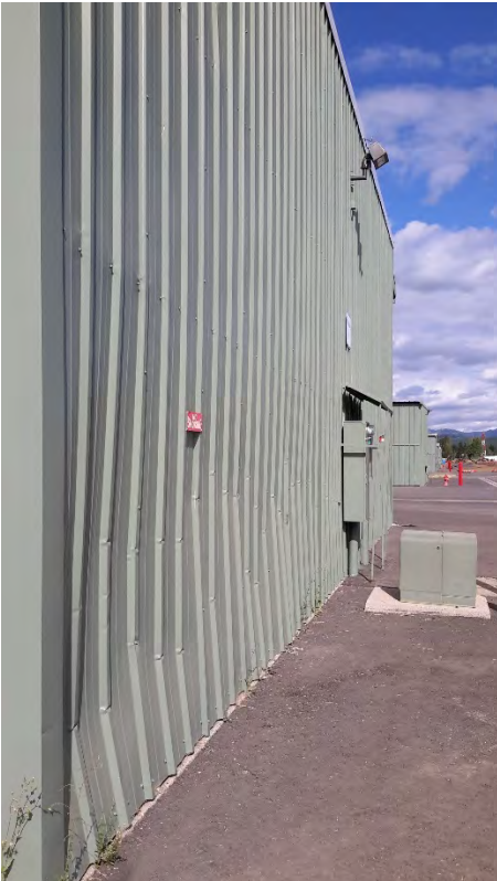
Figure 111 Hangar H - wall panel damage on north end
