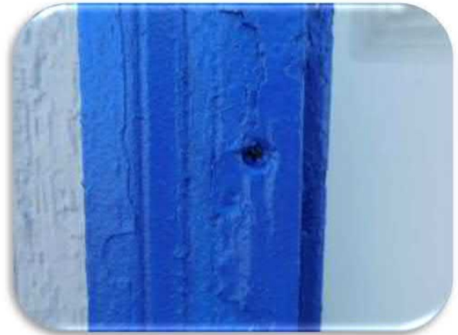
Figure 5-58 shows the typical condition of the siding with lifting paint.
