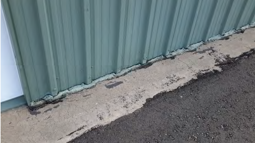
Figure 89 Hangar E - sealant at base of south wall ineffective and will trap moisture against panel base.
