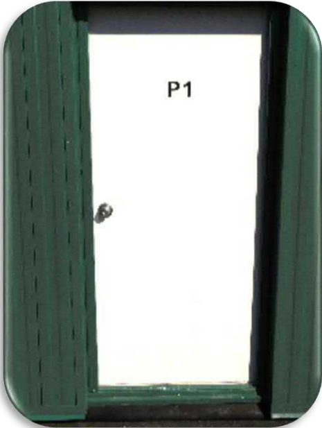
Figure 5-81 shows an example of the condition of the doors on these hangars.
