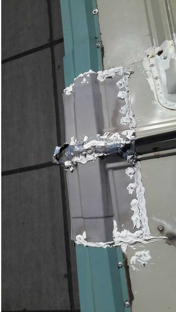
Figure 139 Hangar M - foil and heavy sealant use to try and fix leaks
