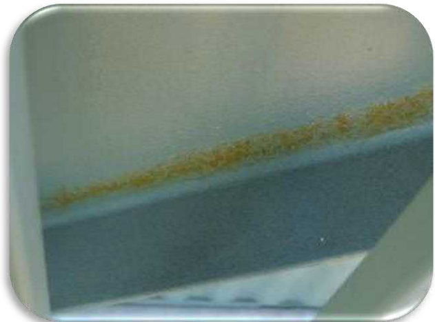
Figure 5-63 shows the typical corrosion on the Air Traffic Control Tower.
