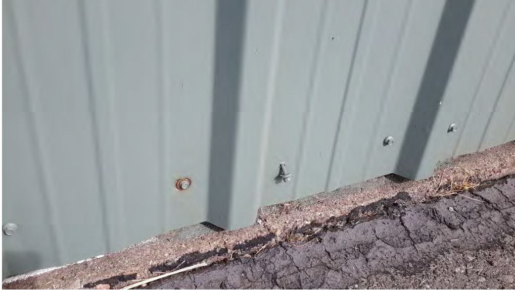
Figure 114 Hangar H - east side panel fasteners show signs of rust and are loose
