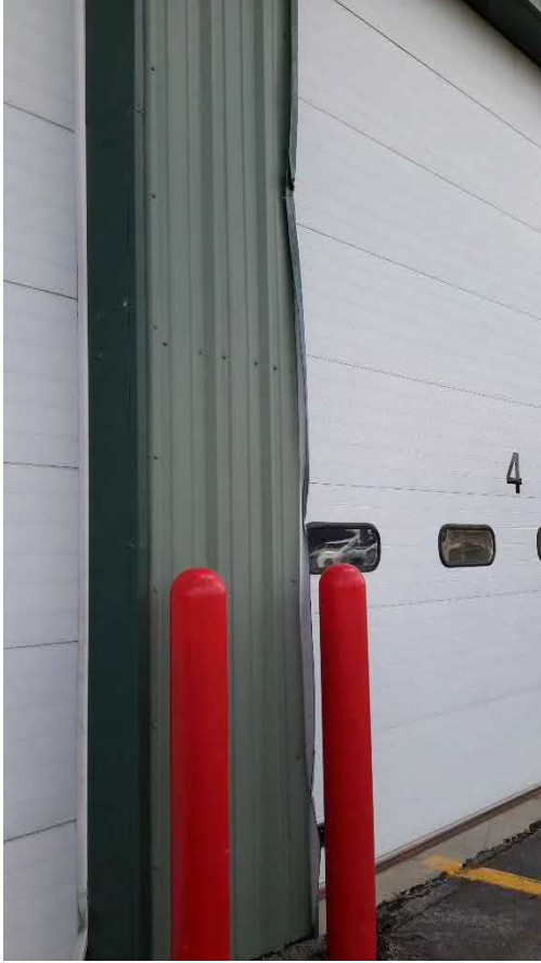
Figure 16 Building 7 - door jamb trim damaged - west side
