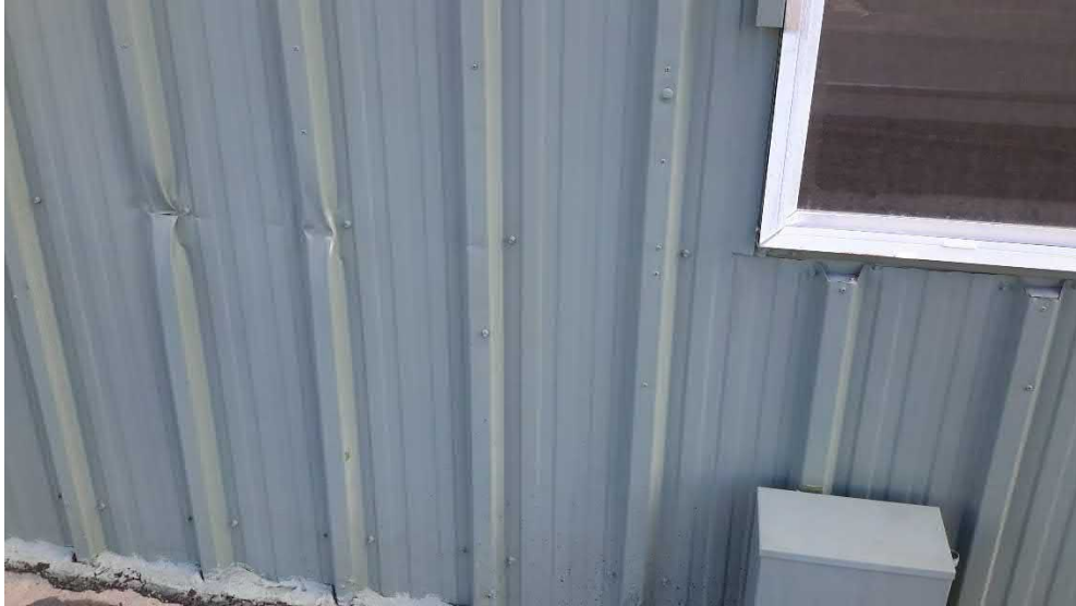
Figure 91 Hangar E - south wall window trim missing, wall panel damage
