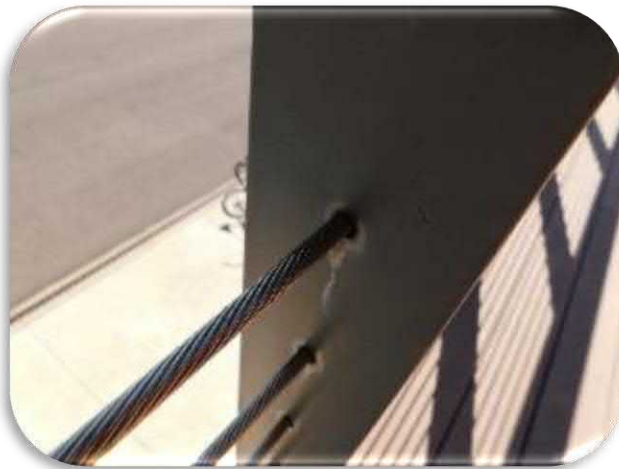
Figure 5-12 shows the mid corrosion that is occurring in the second floor railing post holes.
