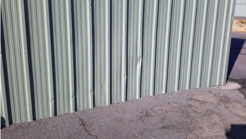
Figure 64 Hangar B - wall panel damage on north end from snow and ice
