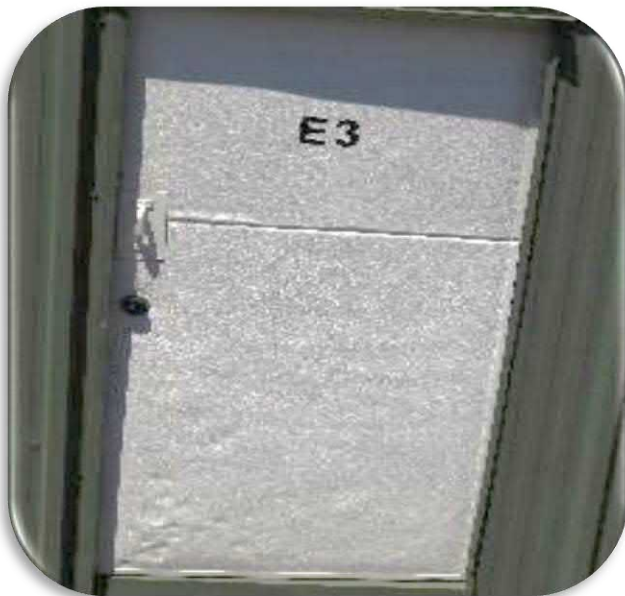
Figure 5-75 shows an example of the condition of the doors. The coating is glossy, but the door is damaged
