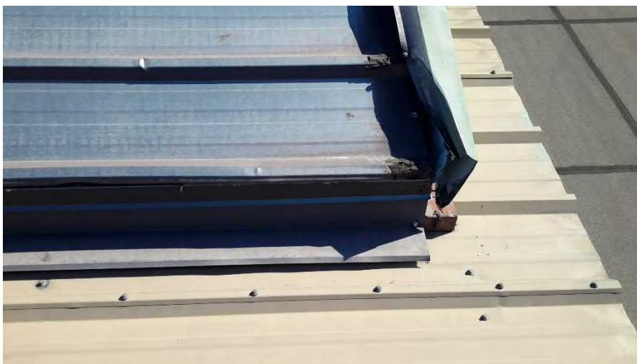
Figure 55 Hangar A - damage to roofing / trim at over-frame area, south east corner
