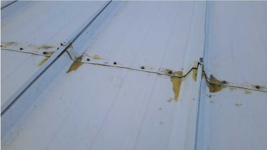
Figure 106 Hangar H - screws missing and loose at midline lap joint
