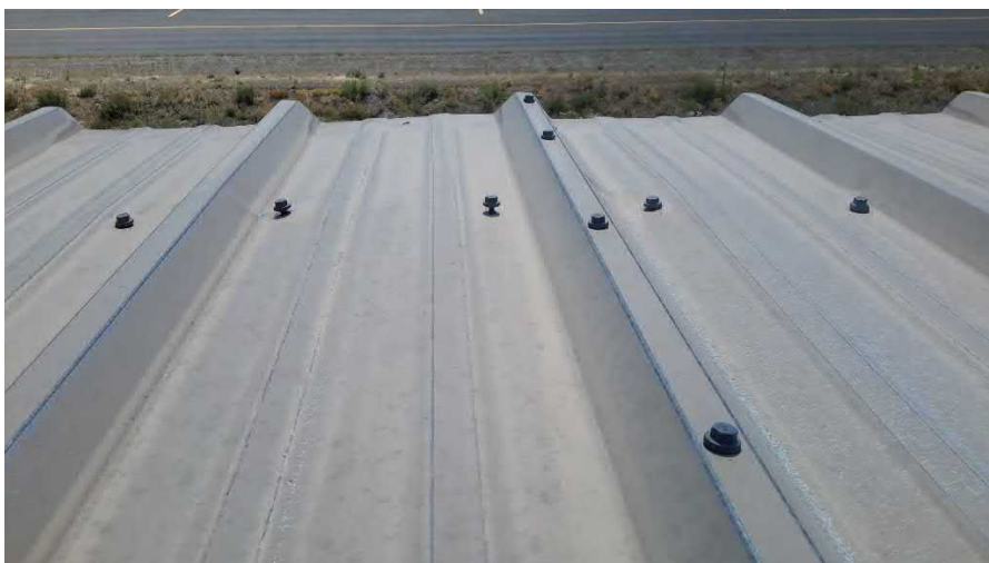
Figure 95 Hangar F - loose screws evident on roof
