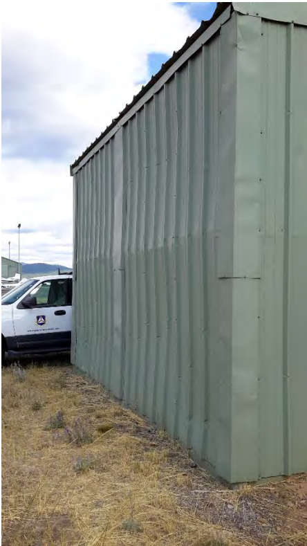
Figure 43 Building 12 - wall panel damage from snow and ice, south side
