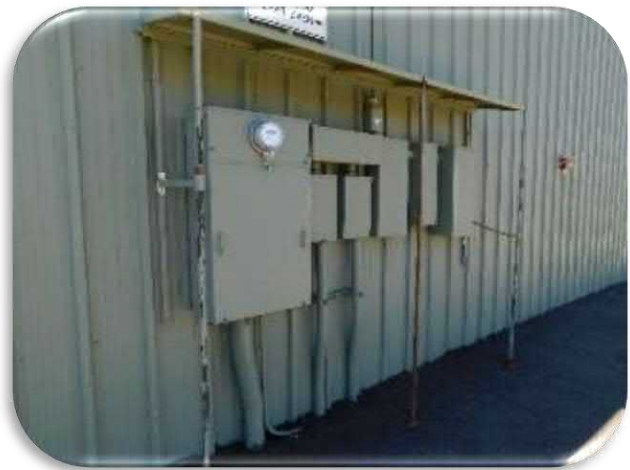
Figure 5-76 shows the rusted and unpainted posts on the electrical equipment canopy.
