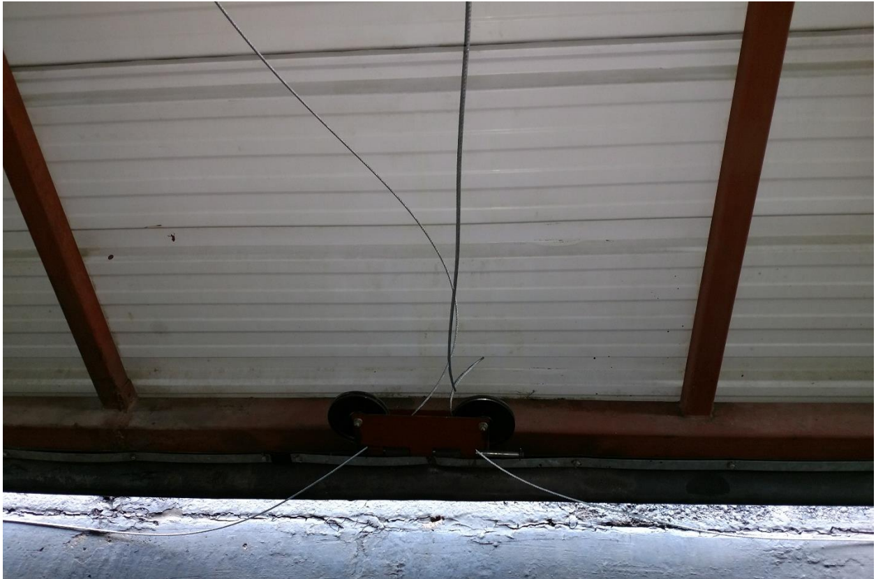
Fully slack cables.
