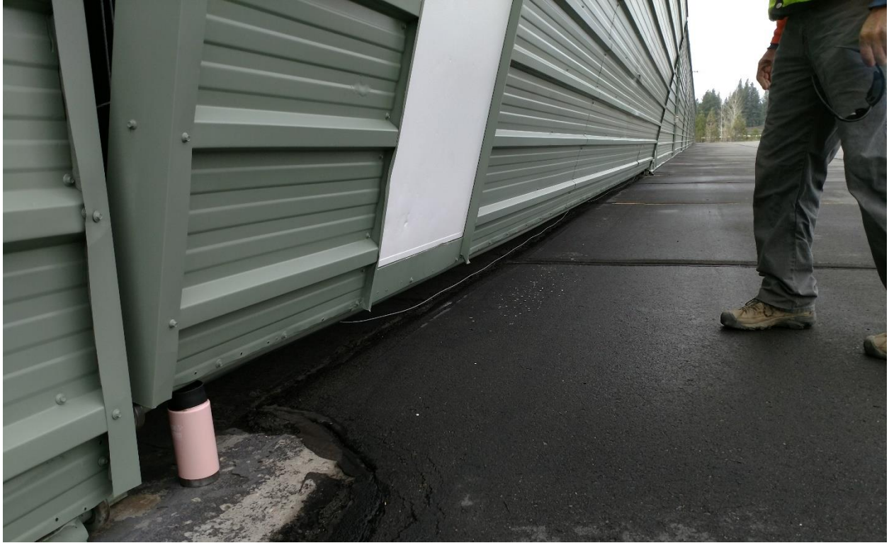
The coffee mug was found holding the entire weight of the hangar door. Slack cables are seen under the hangar door.
