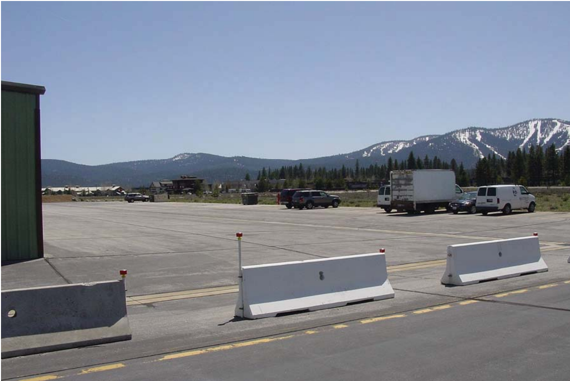
EXISTING PARKING AREA, NO DEFINED ACCESSIBLE PARKING SPACES.
