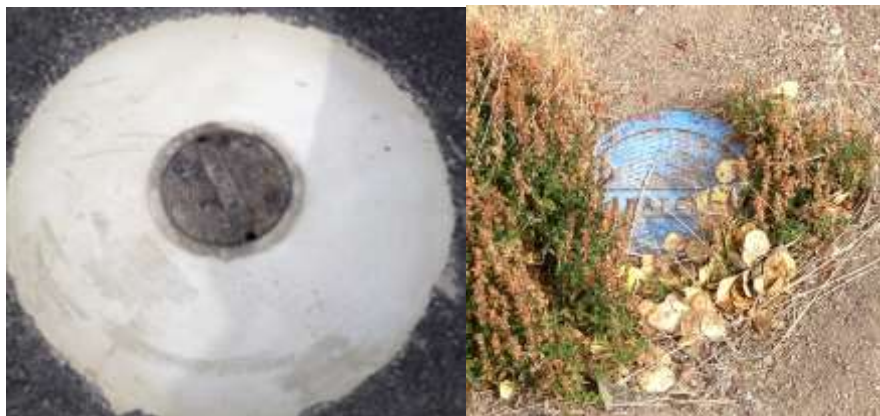
Water System Valves
